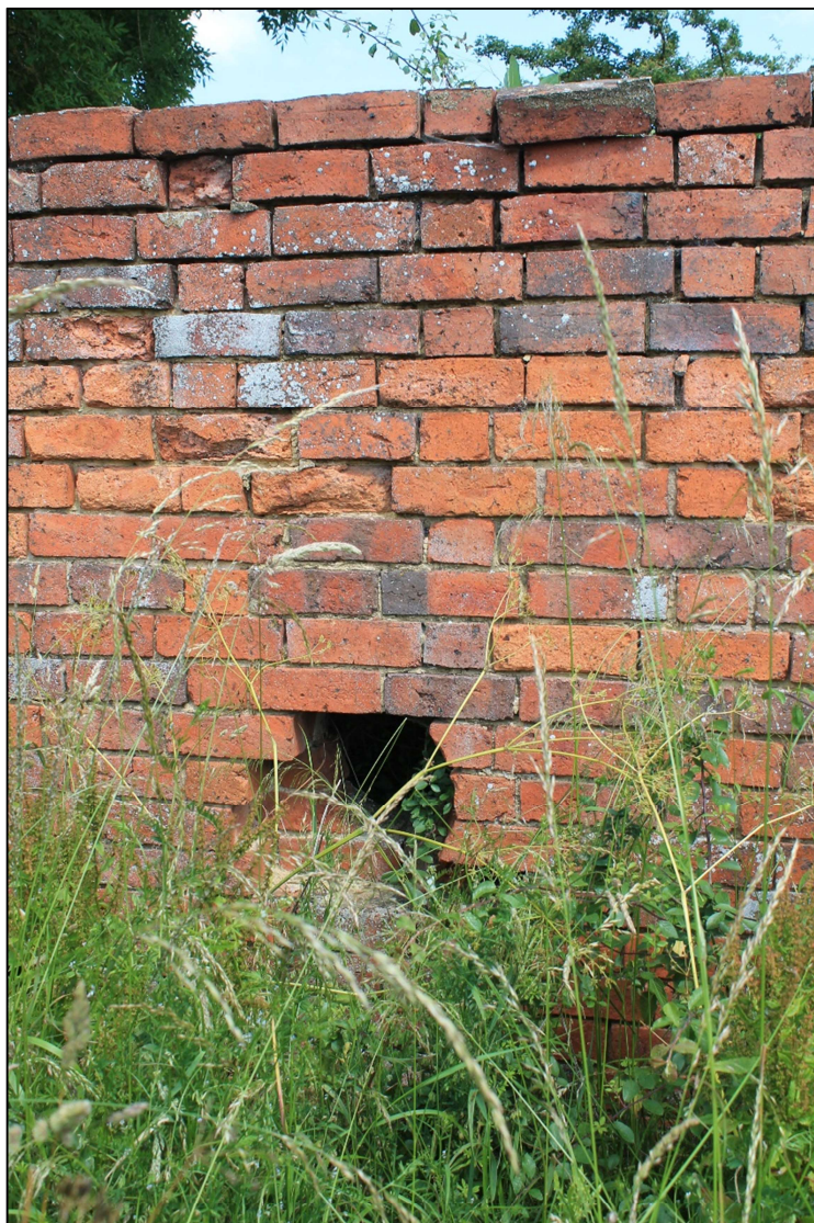
Plate 14 Detail of east wall of cattle yard (Area 6) showing hole through wall, looking northeast
