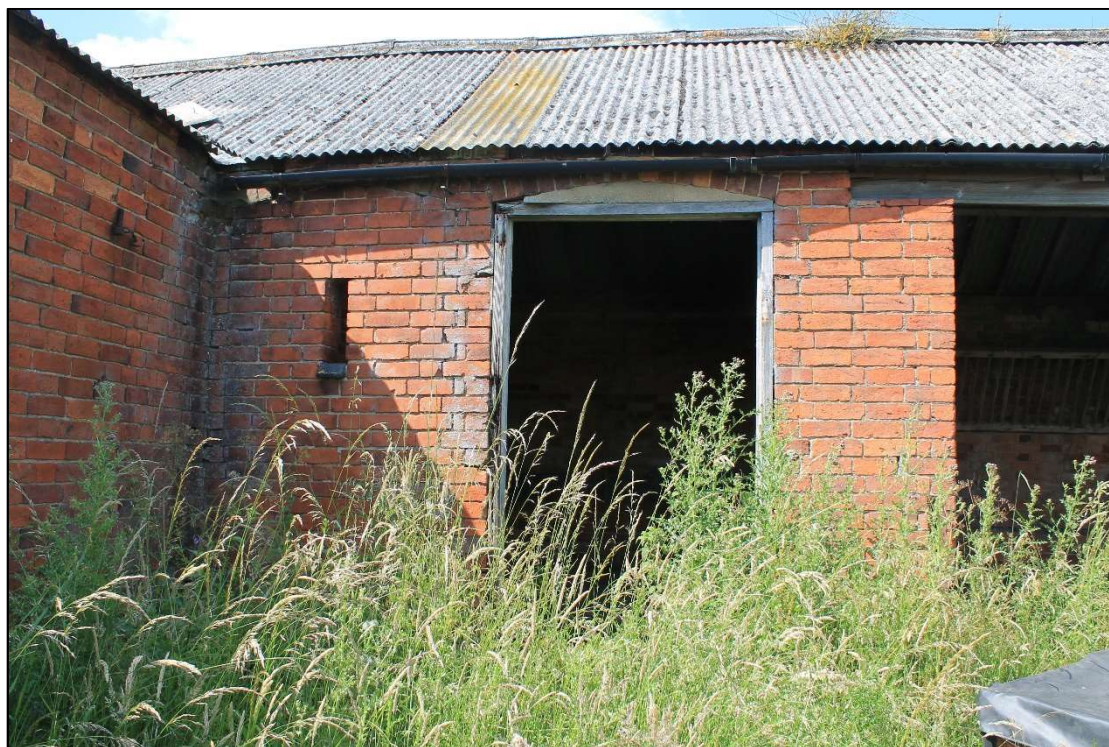
Plate 15 South external elevation of Room 3, showing blocked window and inserted breather slit, looking north
