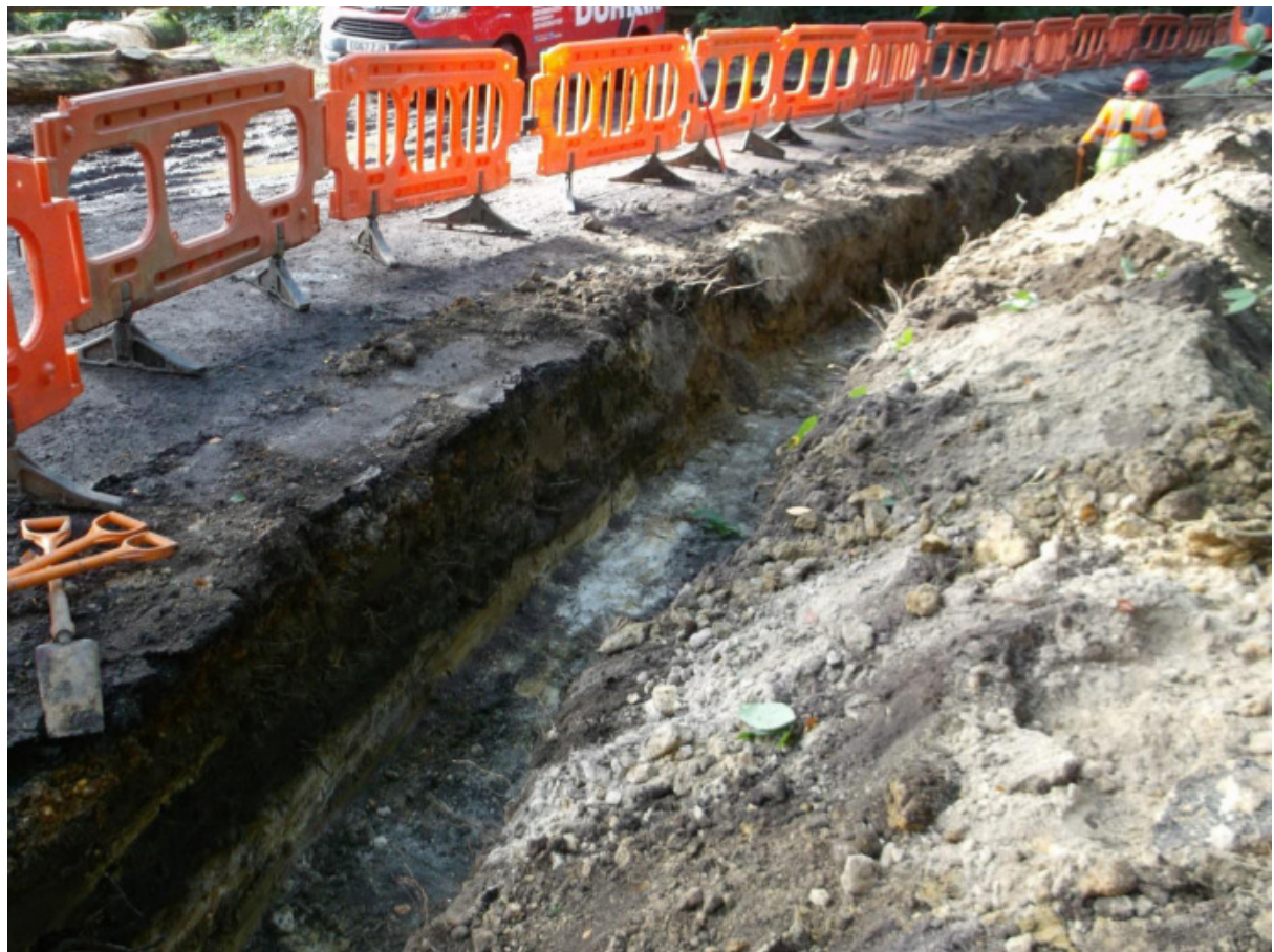
Plate 2: General view of stratigraphy in Area 1 showing modern backfill (105) relating to the existing 132 kV cable trench, looking south
