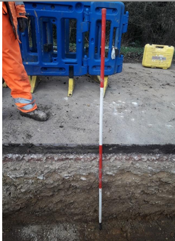
Plate 10: Post-excitation shot of the sewer trench at the south-eastern end of the works showing the stratigraphy looking north-east
