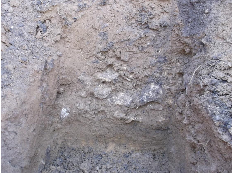
Plate 7: Section Manhole 04 leading to the sewer trench showing what was thought to be the possible Roman road (Akeman Street) looking north-east
