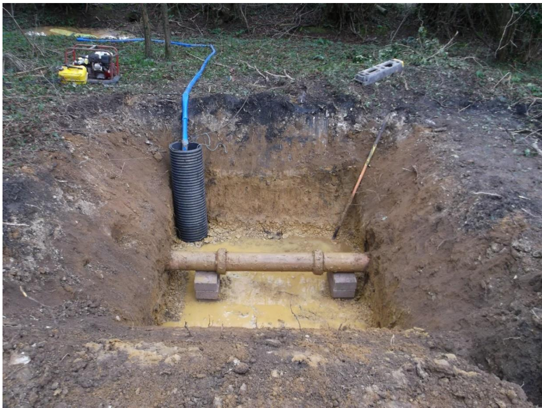
Plate 8: Post-excavation shot of Manhole 04 showing stratigraphy and existing sewer pipe looking south-west
