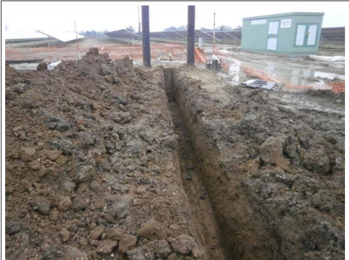
Plate 8: General shot of the new cable trench looking south towards Trench 1 and the new H pole.
