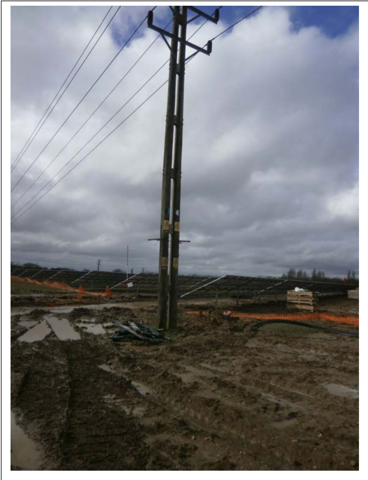
Plate 1: General shot of pole P33854 and the unfinished cable trench within the solar farm development looking west-north-west.
