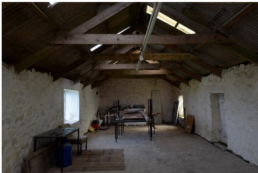
Figure 14: Looking east into the first floor of the stables. Note the concrete lintel above the window in the north elevation indicating its modern date and the loading door to right.
