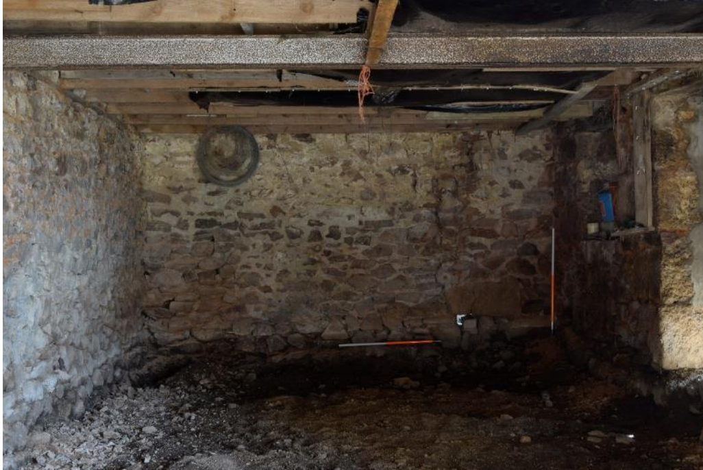
Figure 13: The east end of the stable, showing the dug out interior floor, limewashed walls and a drain hole (bottom right) and details of the iron girders inserted to support the first floor joists.
