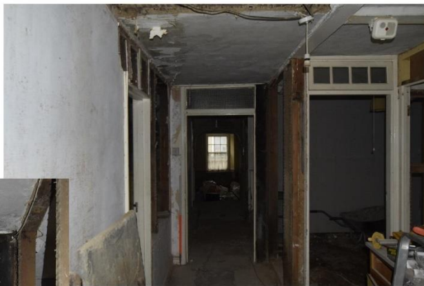
iii) Building 3 Passage way doorway detail. Mouldings are C20 as is glazed panel above.
