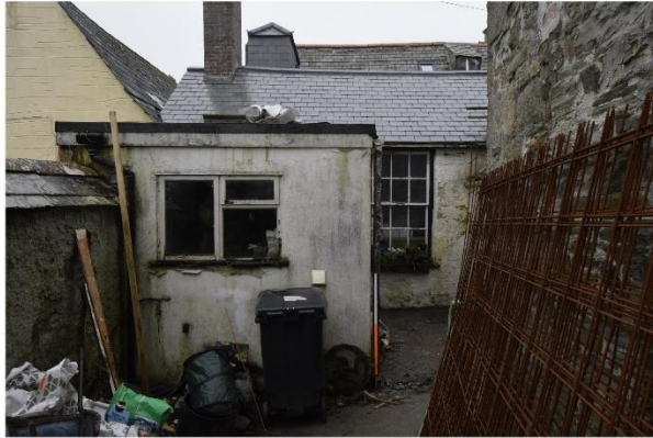
i) Rear Kitchen: NW elevation. Note blockwork construction, modern fenestration and felted flat roof
