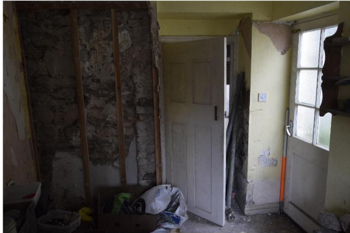
ii) Rear Kitchen: Interior facing SE. Note Early C 20 4 panel door and modern glazed exterior door
