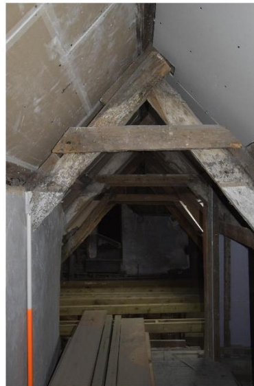
Figure 13 8 Bank Street St Columb Major Building 1 Attic space and roof trusses Copyright Statement Heritage 2018 Images prepared DJR 10/04/2018 Project Code BASC0318
