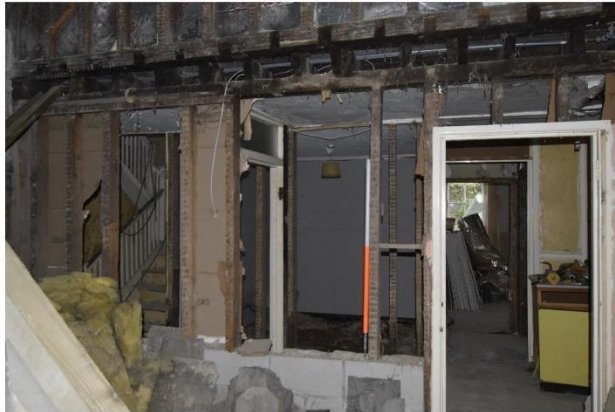
i) Building 3 - Service passage partition. Looking S from Building 4. Note C20 moulding detail around door and existing blockwork under studs
