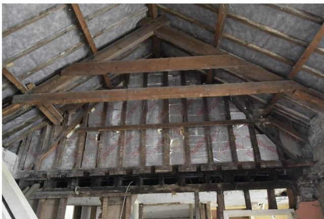
Figure 5 8 Bank Street St Columb Major Building 4 Roof structure Images prepared DJR 10/04/2017 Project Code BASC0318 Copyright Statement Heritage 2017
