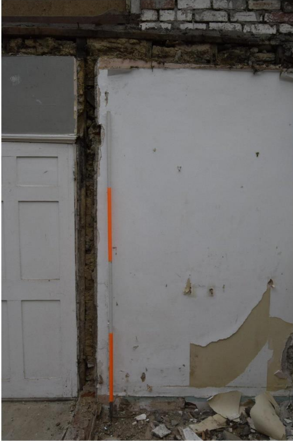
i)(above) Wall D. Timber stud construction with mud and stone infill visible at top where modern ceiling has been removed. Plaster is modern.
