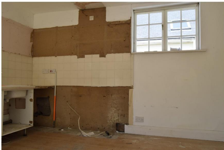
i) NW corner of space consented for demolition. Note exposed modern concrete blockwork to the left of ranging pole
