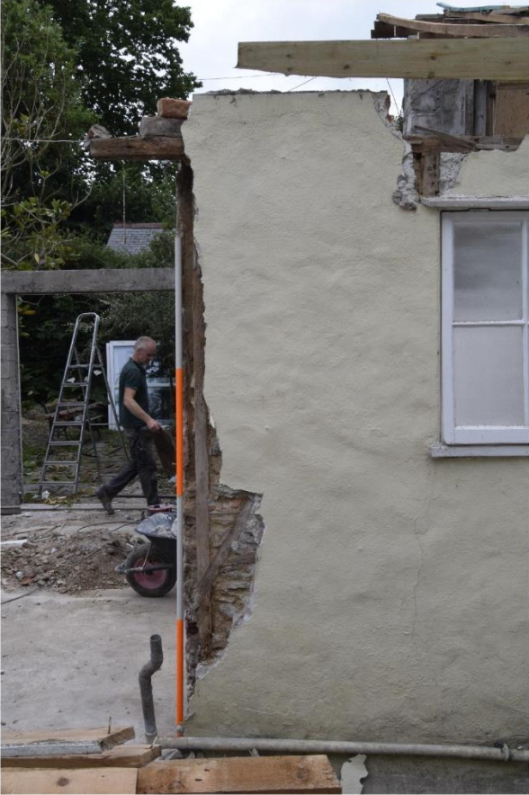
ii)(above) Wall F: Timber and stud construction visible at left-hand side beneath modern cementitious render
