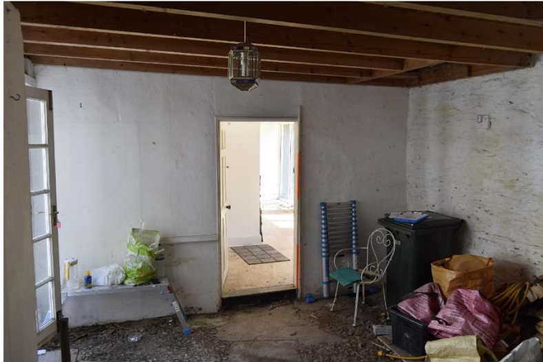
i) Dividing wall 'D' from the SW - - note evidence of older blocked door to left of shot. This wall is of thin stone construction - probably built as a non-supporting internal wall. Doorway is a wide stable-type internal door of early 19th century 6 panel style.
