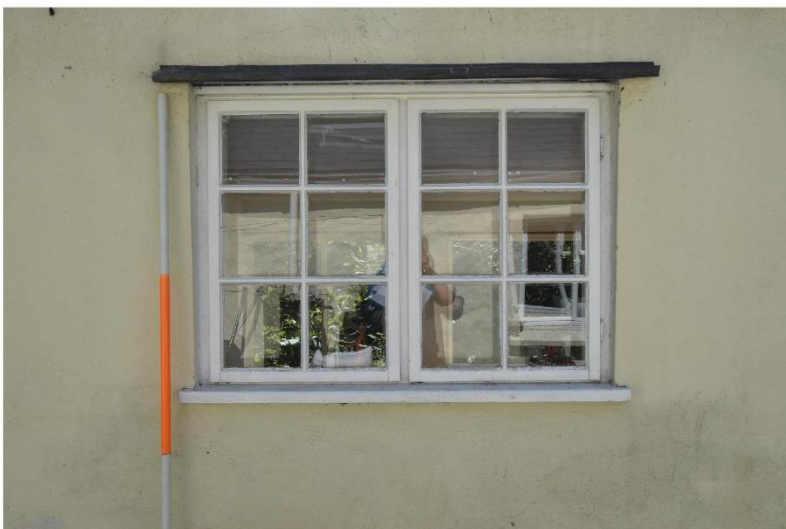
ii) Window 'A' Late 20th century 'weatherseal' type casement. The window has been set across the internal wall. Note cast iron rain hopper and downpipe to be retained (outside consented area).
