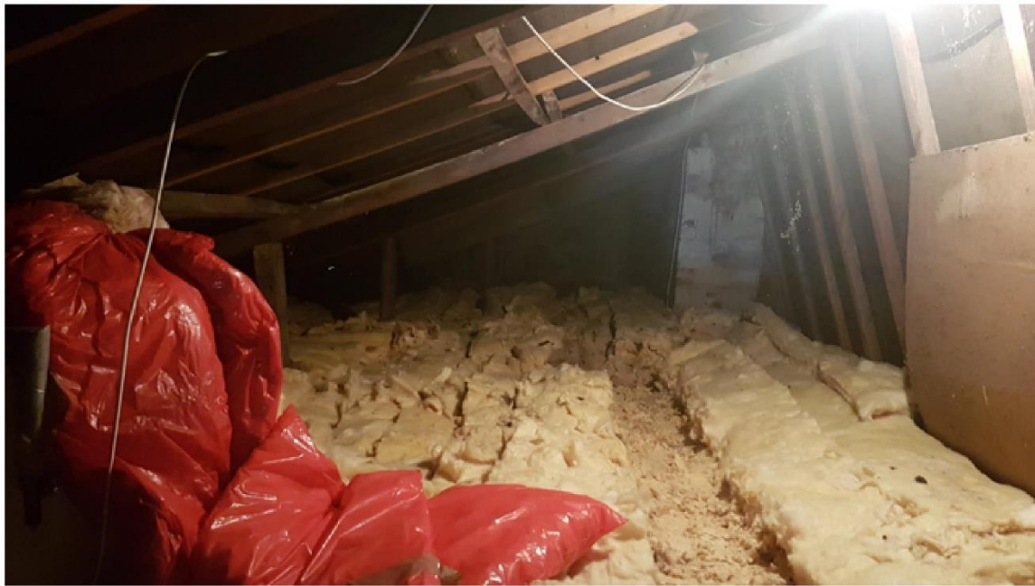
i) Interior of roof to be demolished looking NE. The roof structure is of entirely modern common rafter construction. The modern weatherboarding above the patio doors is to the right of shot. Behind is the top of historic stone wall 'E' which appears to be neatly quoined indicating that this wall always terminated at this point.
