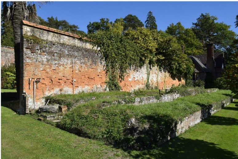
ii) Terrace B looking east - note decayed brick facing
