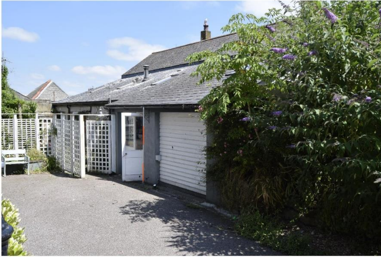
i) Outbuildings - NW elevation from south. Two conjoined lean-to ranges under fibre cement roof coverings
