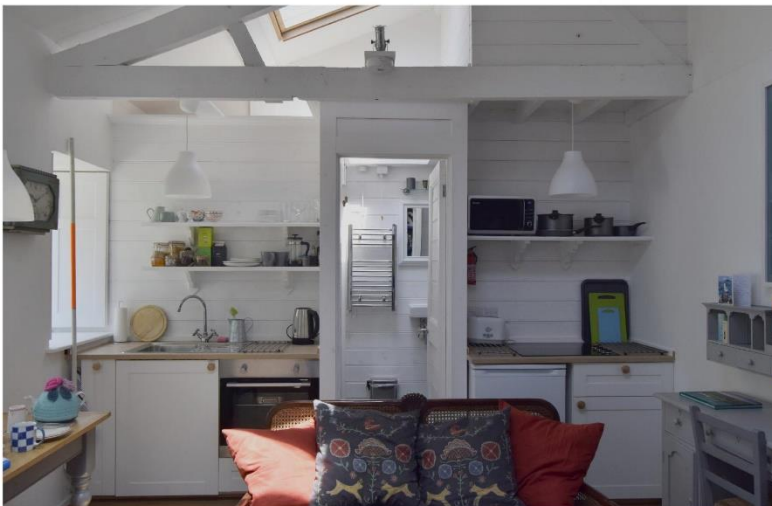
ii) A simple boarded timber screen has been inserted in order to form a modest bathroom in the north end of the building, against which a small kitchen has been fitted.
