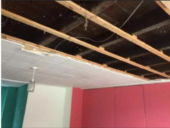
i) showing that the ceiling removed consisted of modern plasterboard, covered in places in polystyrene, fitted over modern battens. Historic timbers behind
