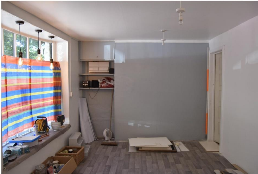
i) looking north through the main 'shop' space - note stud wall to the right of shot.
