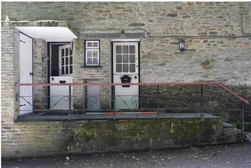
ii) detail of 1960s alterations to northern elevation facilitating separate access to shop and flat
