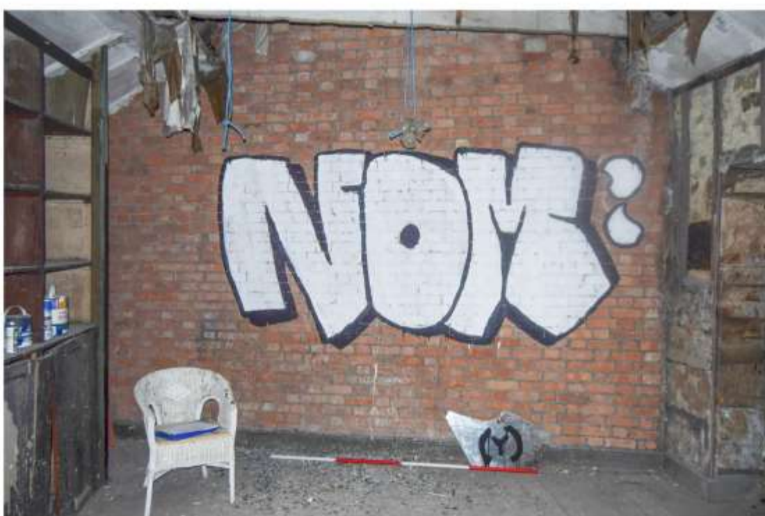
iv) North wall. Brush painted graffiti dates to 2020-2022 LLOY1022_0301.jpg 2m scale
