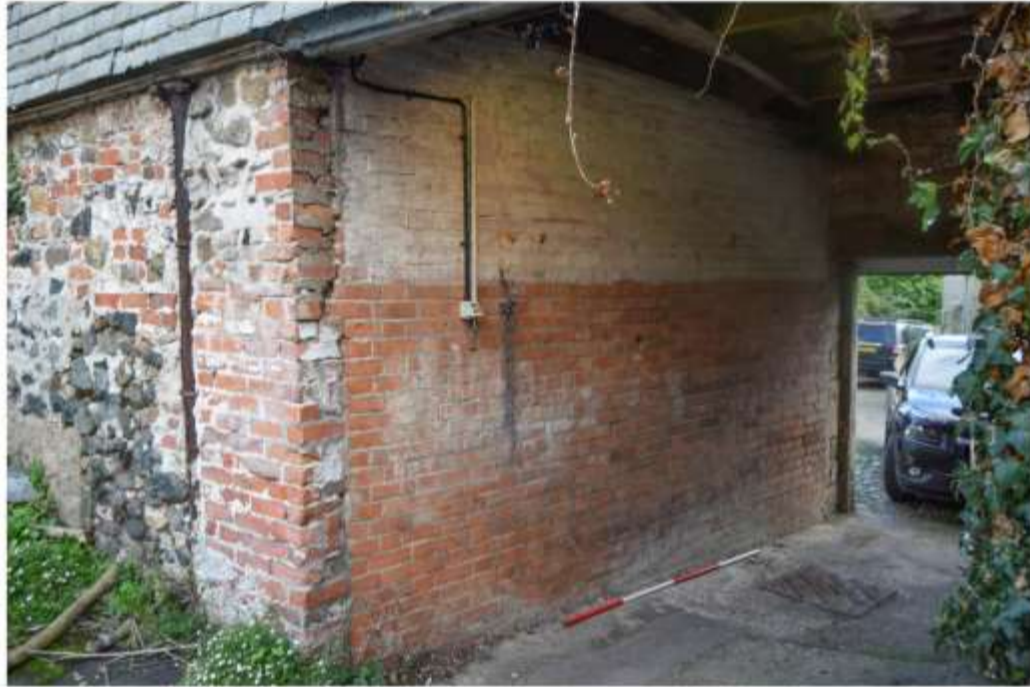
iii) North wall of Space 1. This wall represents 'Phase 3' infill - demonstratable with reference to its constructional material of pressed 'Fletton' brick within cement mortar.
