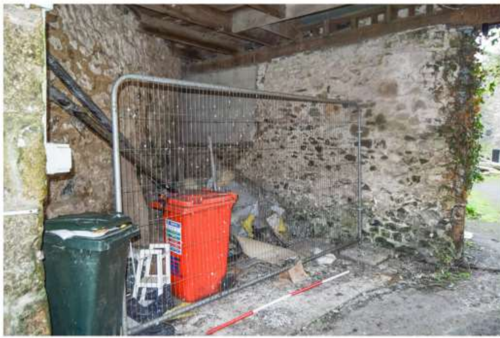
i) Looking southwest into Space 1. The wall to left is stone rubble, likely the Phase 1 plot boundary, the wall to right is rubble infill between the iron pipe uprights of the west elevation of the east range. The concrete block infill panel corresponds to slate hanging over lath within Space 2.
