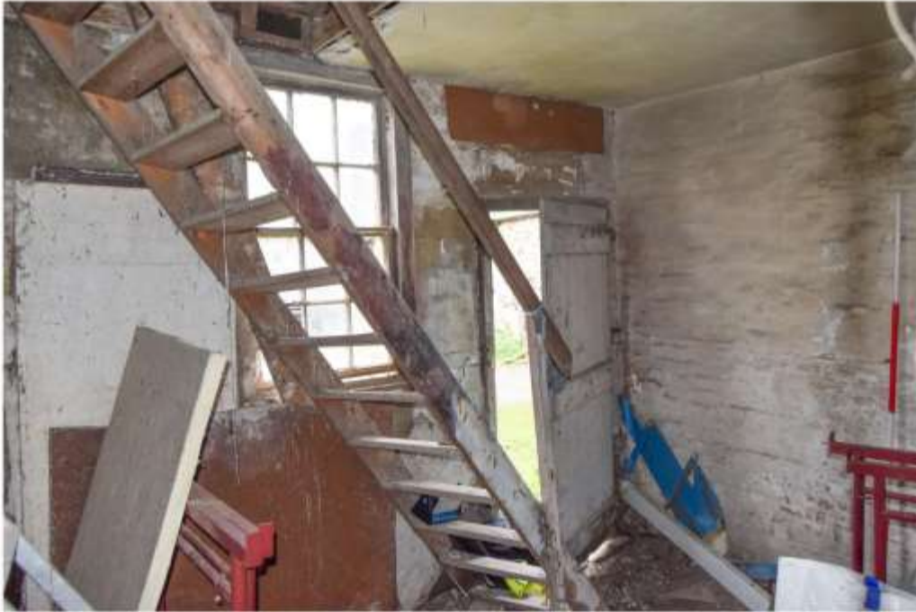
ii) north and east walls of Space 2, both of brick. the simple stair is considered relocated to this location, possibly from Space 1
