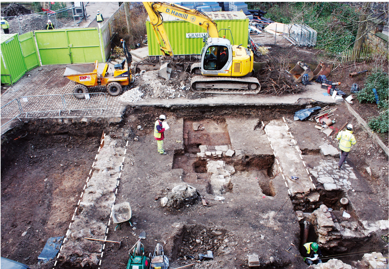
Illus 37 General view of the remaining Royal High School walls (C042 and C054), facing west
