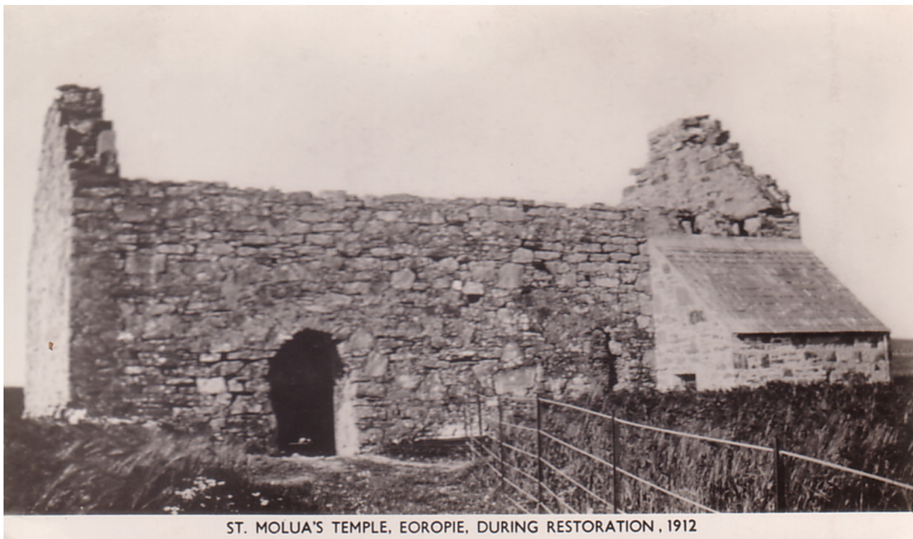
Illus 5 Postcard of 'St Molua's temple, Eoropie, during restoration, 1912' (reproduced with kind permission of Comunn Eachdraidh Nis)
