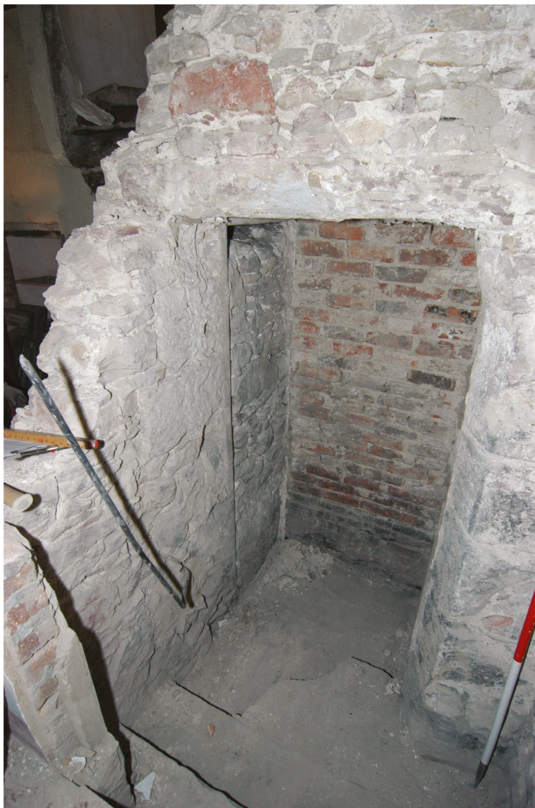
Illus 35 Blocked doorway in Room S07 with chamfered door surround. (© CFA Archaeology Ltd)
