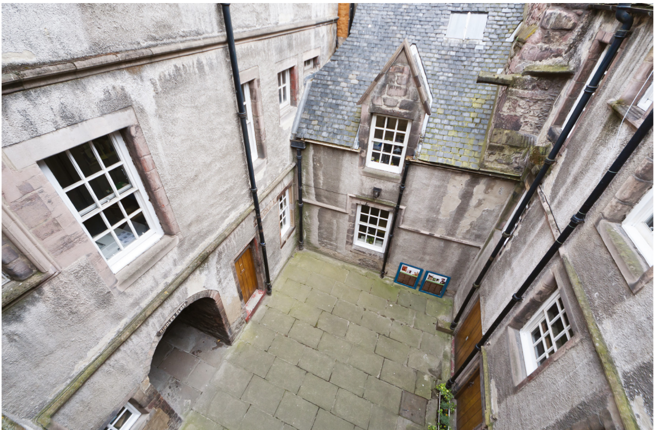
Illus 13 View of the courtyard prior to alteration works. (© Scottish Historic Buildings Trust)
