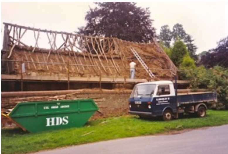
Fig. 20 From the road showing the thatch removed and the original roof timbers exposed (most of these were replaced).
