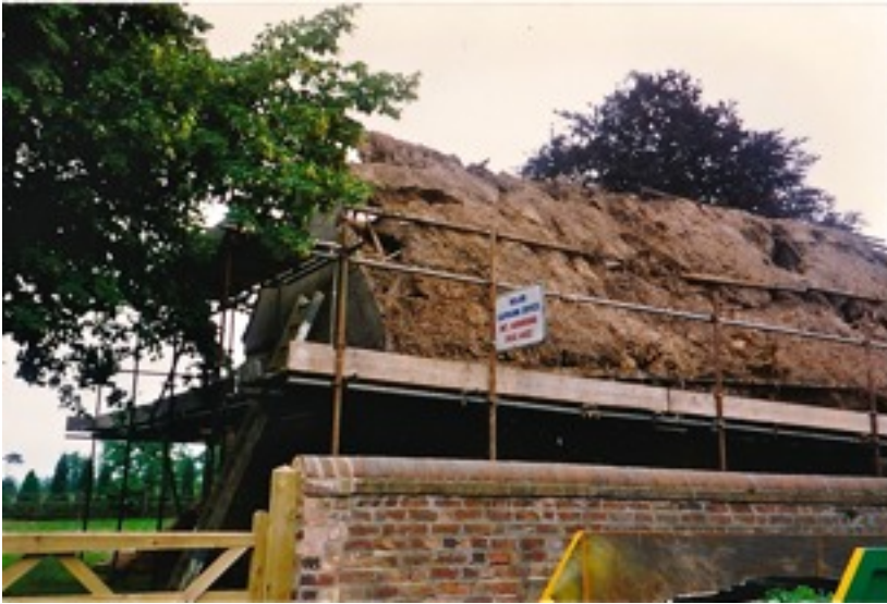
Fig 18. From the road showing the remains of the thatched roof below the corrugated iron.
