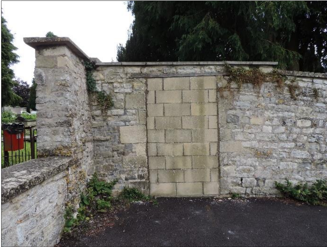
Photo 3: Blocked doorway from original path
