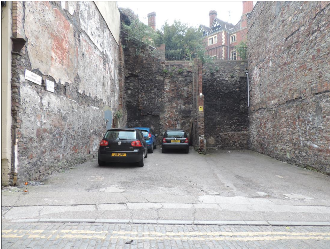
Photo 6 South-eastern boundary wall to the Project Site. Clearly once part of an earlier structure.
