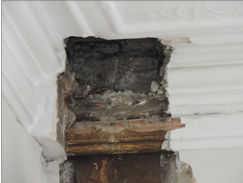
Photo 11 Detail of altered cornice with wooden baton addition to the base.
