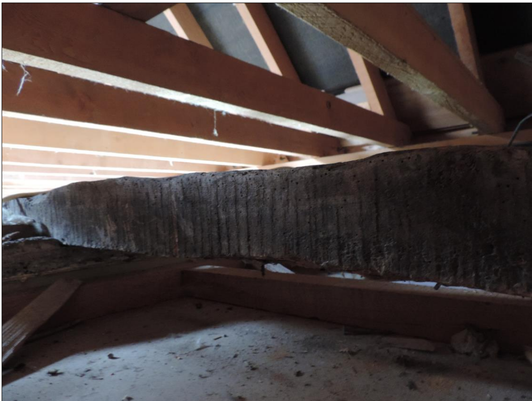
Photo 6 Detail of floor joist resting on the top of the partition wall
