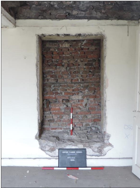
Photo 2 c. 1790 / 1800 Southeast bricked up window, northeast facing view (Scale 1 x 1m & 1 x 500mm).
