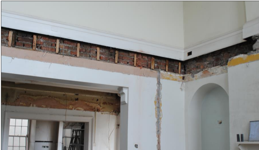
Photo 14 East facing view of brickwork revealed following the removal of the floor joists.
