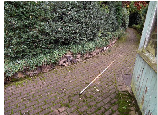
Photo 8. The low retaining wall opposite the garden sheds, looking south. Scale 2m.
