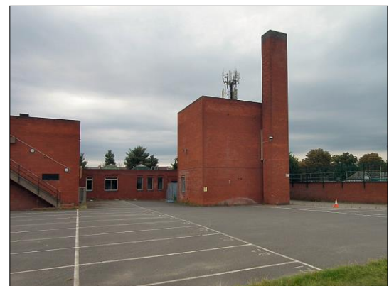
Photo 3. Block 1 with chimney, and part of the eastern face of Block A, looking west.
