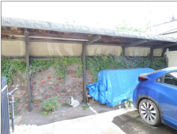
Photo 2 Section of lean-to extending from the single storey modern extension to 7 Richmond Hill Avenue (NNE facing view)
