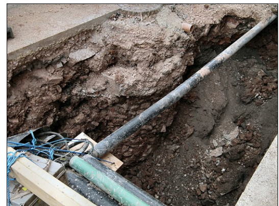
Photo i. Exterior of the well as exposed in the northern section of the trench, looking northeast.
