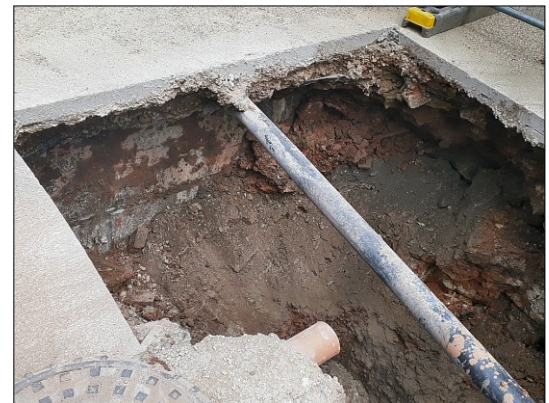
Photo k. The eastern end of the trench, looking southeast, showing the western wall of the underground boiler room.
