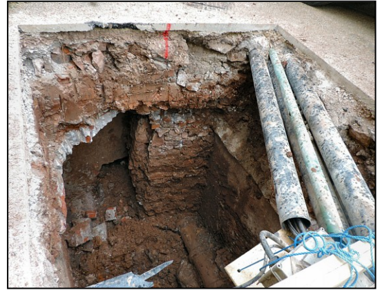
Photo d. View of the chamber after excavation and removal of vertical pipe, looking west.
