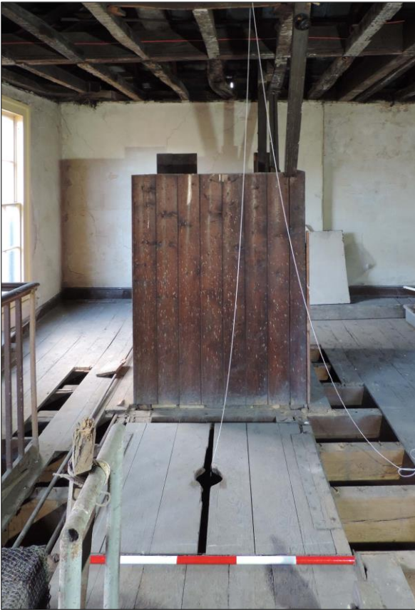
Photo 6 Southeast facing view of hatch and shaft in the background. Scale 1m.
