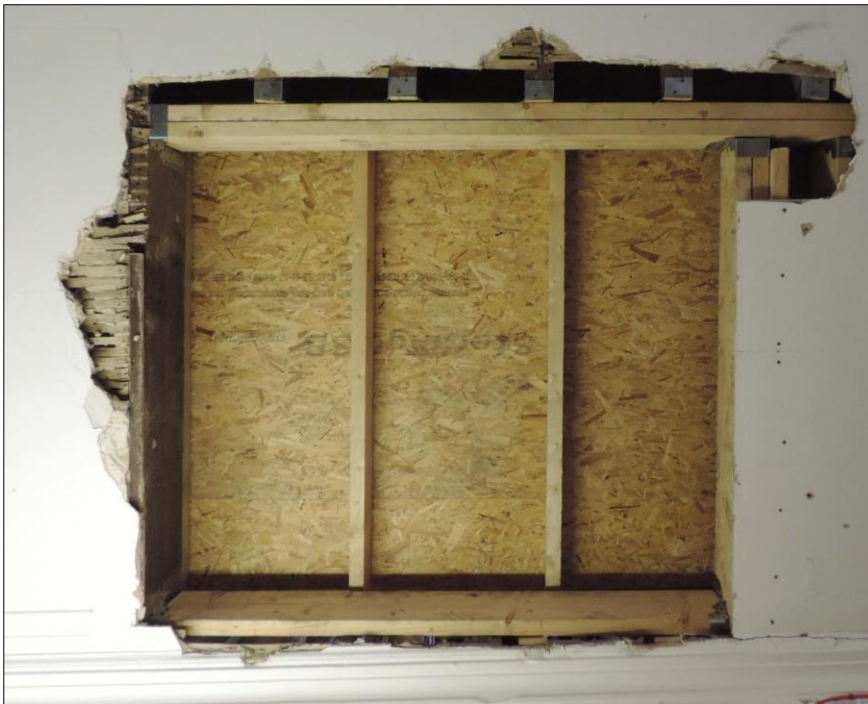
Photo 8 View of underside of Second Floor cut, taken from the First Floor. 19 th century lathes visible against the northwest and southwest of the cut.
