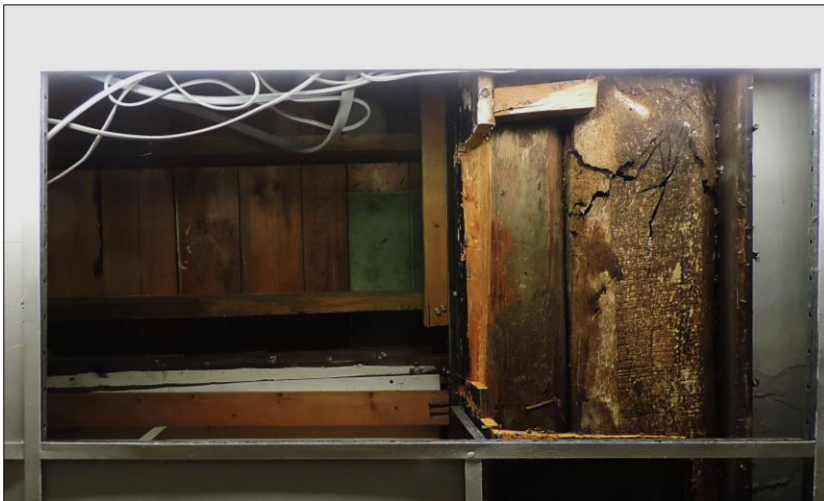
Photo 2 Partially exposed section of northwest-southeast potential 18 th century floor beam, supporting the First Floor joists. Photographed from Ground Floor level.
