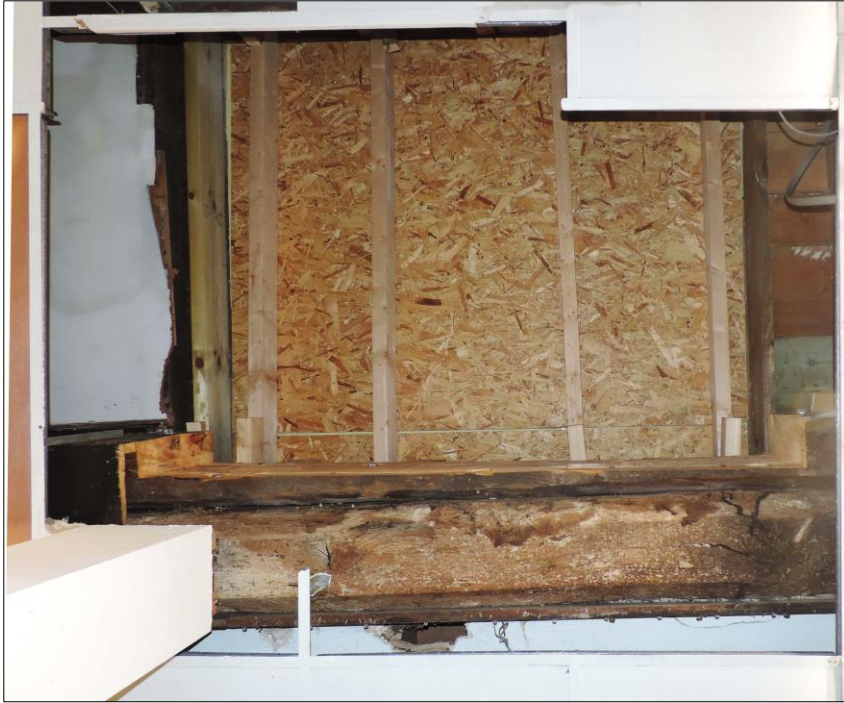
Photo 3 Section of potential 18 th century beam exposed after cutting of new lift shaft.
