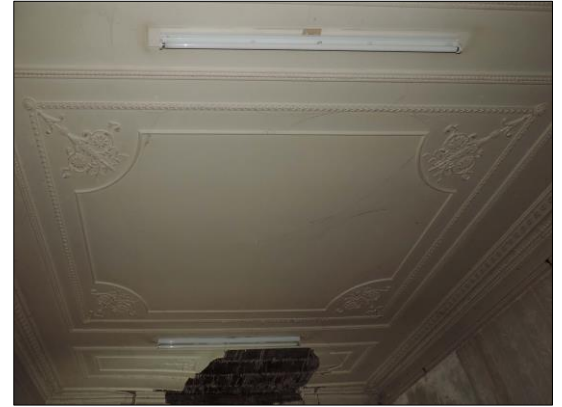
Photo 12 View of Room C ceiling looking towards the bay window and water damage to plasterwork.
