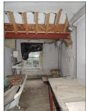
Photo 26 northwest facing view of second storey room. Looking out over the front courtyard.
