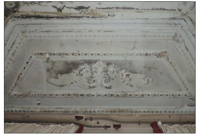
Photo 13 Water damage to plasterwork above cantilever bay window in the rear Family Room (Room D).
