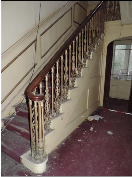
Photo 16 staircase comprising cast iron balusters, polished hardwood handrail, finished at the base with a curtail step
