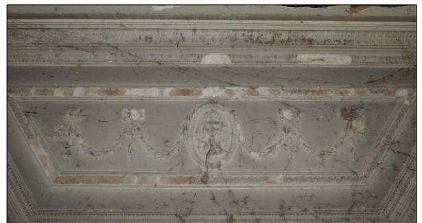
Photo 11 Ornate plasterwork above cantilever bay window in the rear Drawing Room (Room C).
