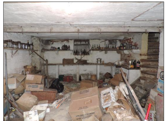
Photo 18 Southeast facing view of cellar with stairs to Kitchen to the left of shot.
