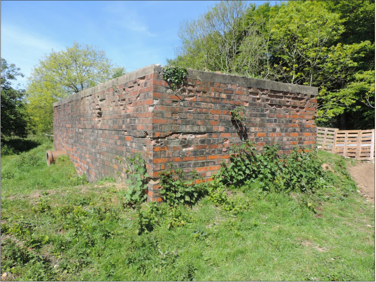
Photo 3 Northwest facing view of the Bunker showing stress to southeast corner.
