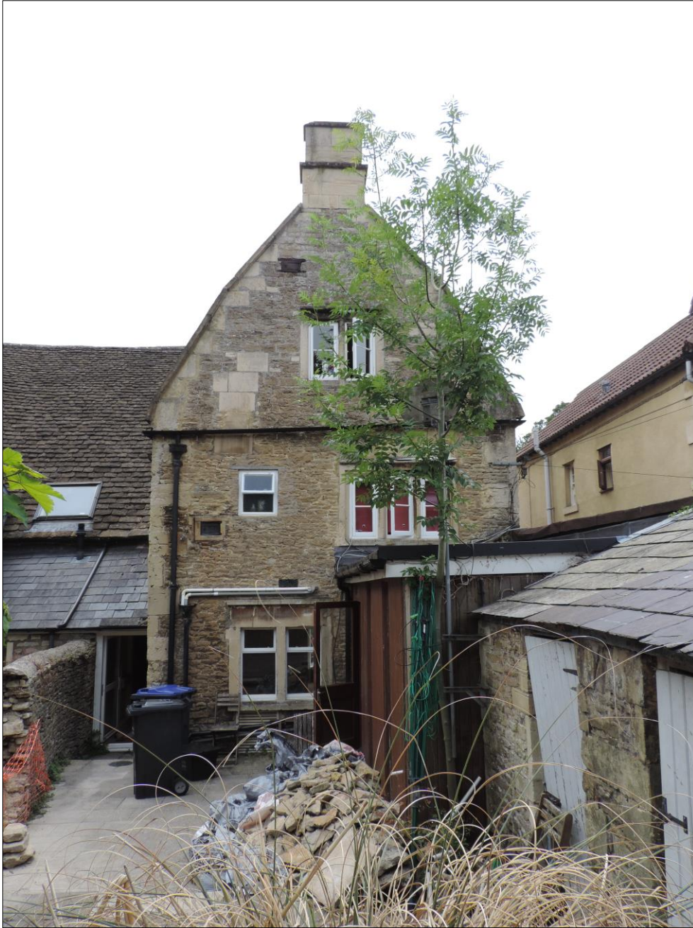
Photo 9 Southeast facing view of rear elevation. Chimney doors are visible to the north of the elevation and a modern bathroom window has been inserted close to the line of the flue. Modern timber annex and outbuildings are visible to bottom right of the photo.
