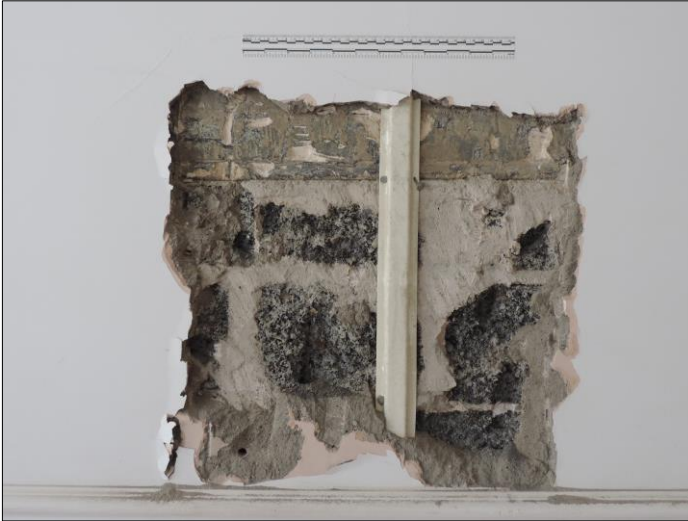
Photo 3 Blocked fireplace in Entrance Room (scale 300mm)
