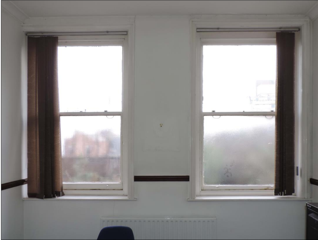
Photo 7 Period window frames. Example to the left of the photo has been partially concealed behind a modern partition.
