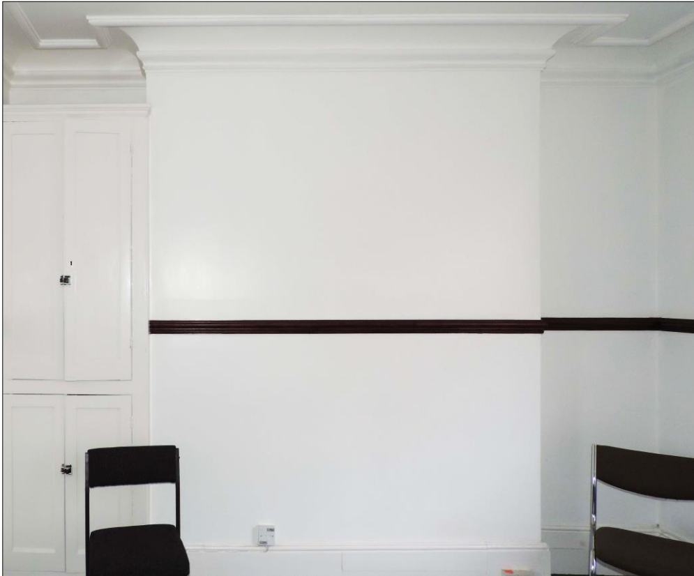
Photo 4 Concealed fireplace with modern dado rail. Cornice above would appear to preserve the 19 th century detail.
