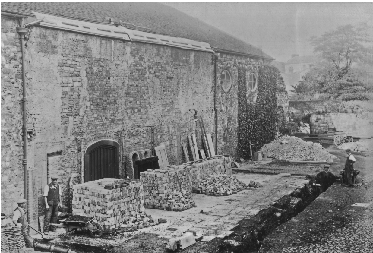
Figure 9.10: The south side of the Great Hall in October 1931 following the demolition of the Grand Jury Room. The foundations for the Entrance Block are being dug. Door 163 is visible on the left, behind the worker with the wheelbarrow and Door 216 is to the centre by the ladder. An infilled oval window (435) is visible above. SANHS 12250.
