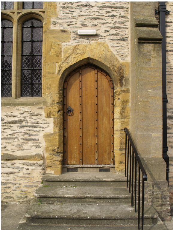
Figure 16.6: Door 512, the south entrance to the schoolroom, showing the reduced ground level and modern buttress.
