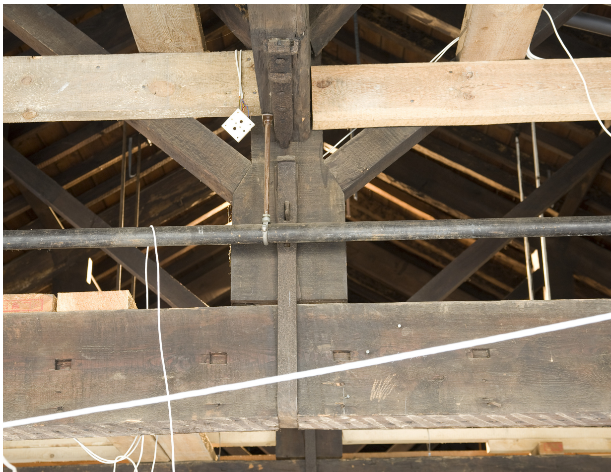
Figure 9.7: Great Hall roof truss 1 from the east, showing the mortices for the ceiling battens, the iron bands holding the joints and the beam linking to the top of Window 101 to support the hipped roof. The pale timbers are all modern additions.
