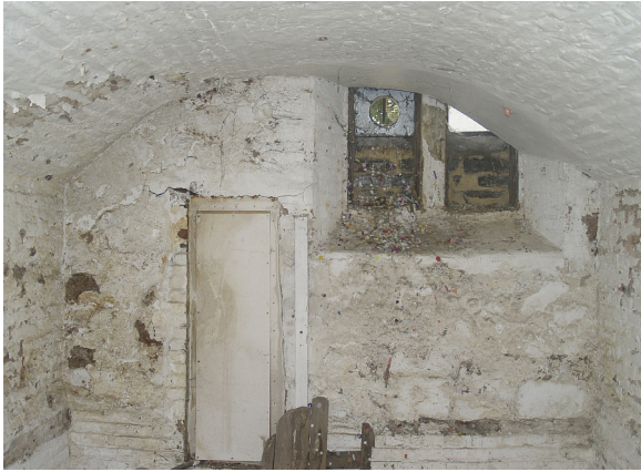
Figure 16.8: The south wall of the cellar with the half-blocked window and access to service pipe.
