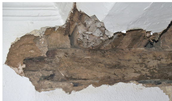
Figure 13.10: Timber, probably from Frame 8 of the 1482 roof with a tenon for an angled joint to the left, reused to form a pad for a ceiling beam in Room 113. TCB10-41.
