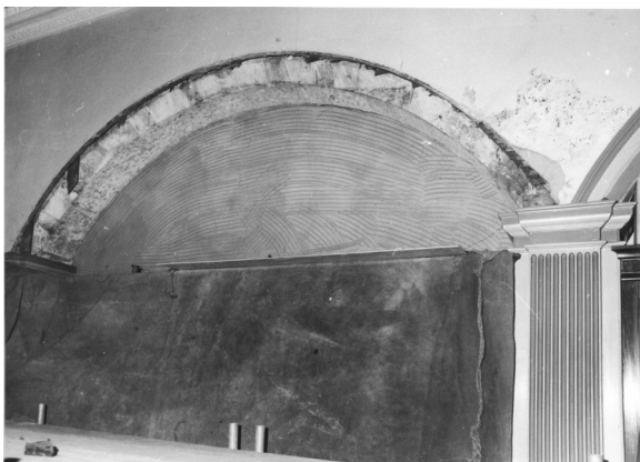
Figure 11.4: The blind arcading in the Adam Library during repairs, probably in the 1970s. SANHS Hawtin 2.
