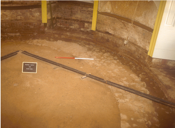
Figure 4.3: The lower room of the Round Tower (Room 46) under repair in 1988, looking south-east with Window 65 to the rear. The thicker medieval wall foundations can be seen as well as the late eighteenth-century brick lining to the walls and window reveals with characteristic embedded horizontal beams. Somerset HER image 53542.
