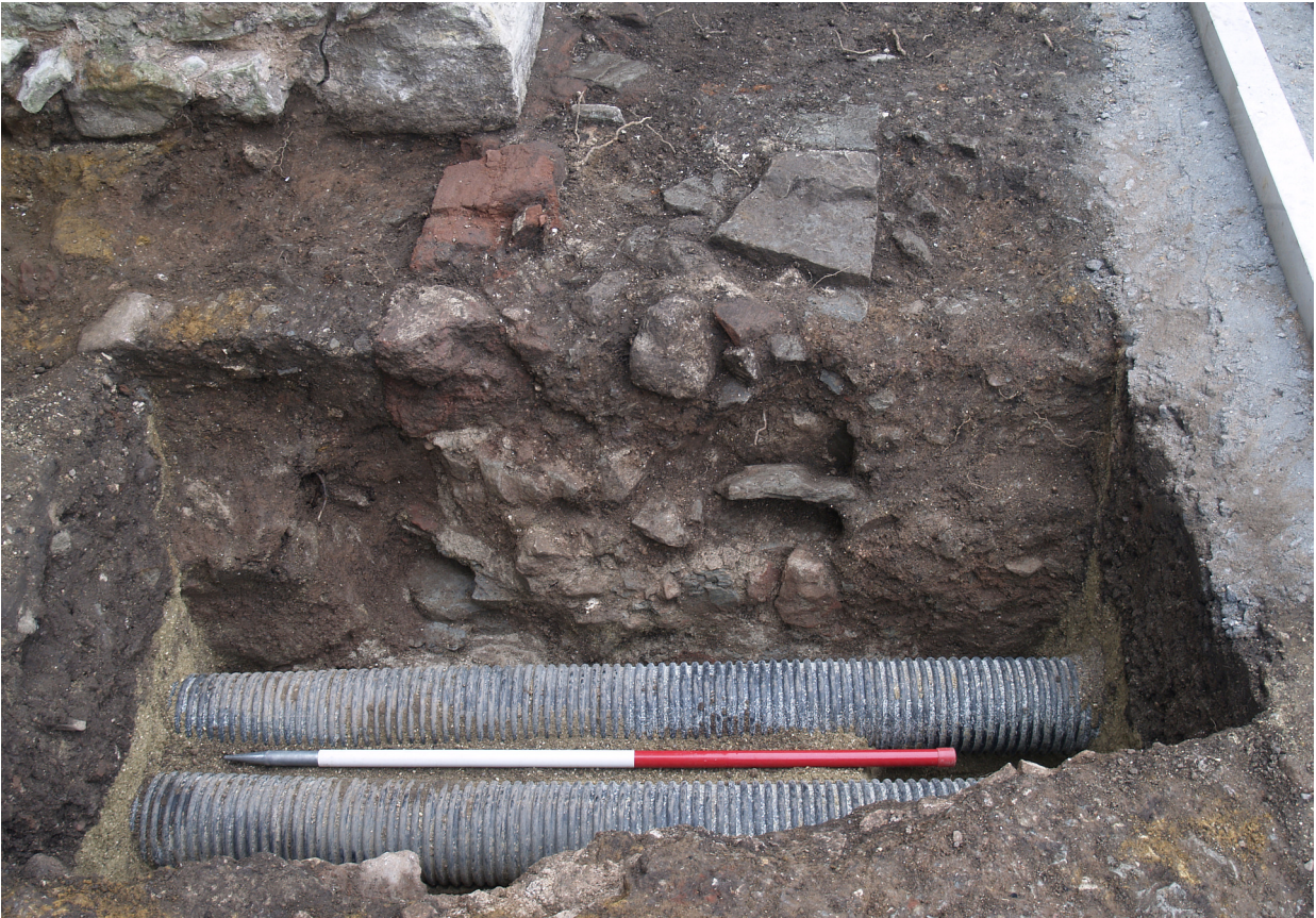
Figure 5.26: Wall 1187 as exposed in the trench for the heating pipes. The red sandstone face is visible to the left just supporting the north wing of Castle House. 1m scale.
