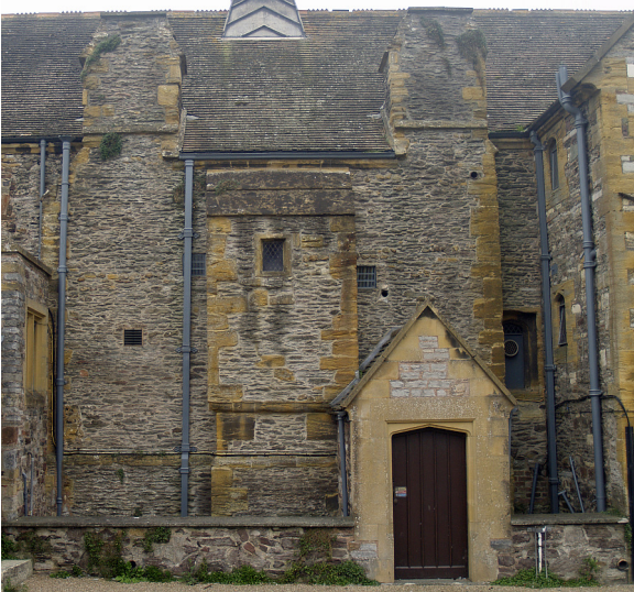
Figure 16.7: The stair and chimney block on the north side of the school. The porch was added over the steps to the cellar in 1931.
