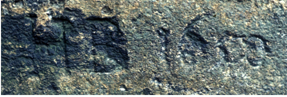
Figure 9.3: Detail of the date carved on Buttress 375 as shown on an undated colour slide. Somerset HER image 30116.
