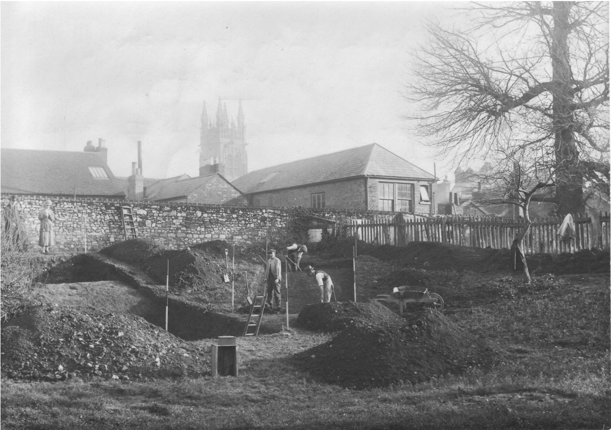
Figure 3.5: Gray's photograph showing the state of work on Friday 5 December 1924. Cutting II is to the left, exposing the marl bank. The men are working in Cutting III which had been started that morning. SANHS 12544.
