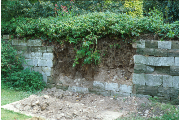
Figure 4.2: The collapsed section of Wall C in 1988. See Figure 4.5 on page 58 for location. Note the lack of solid wall core behind the facing stones. Somerset HER image 29721.
