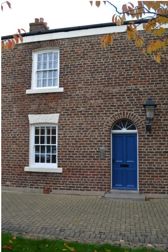
NECT151116TSQ-023 Example detail, external wall (inner elevation on N Range) showing door and windows
