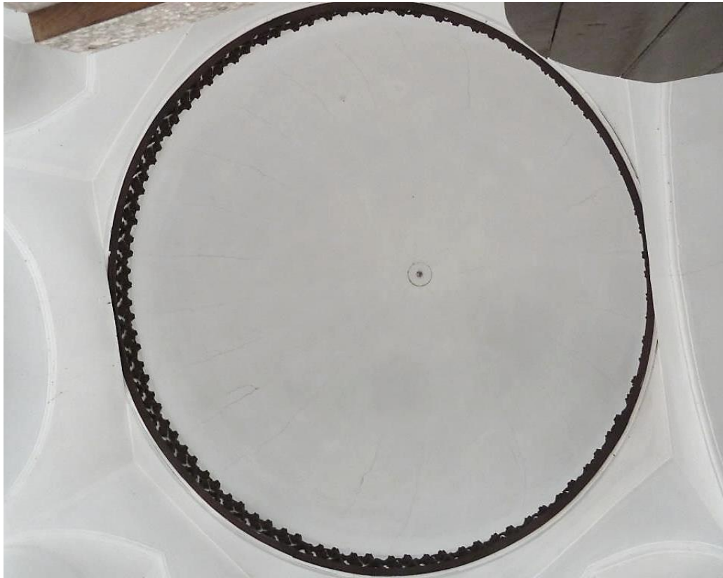
Looking up to plaster ceiling dome & reproduction fibreglass crestring from cast of wooden original in 1979 renovation.
