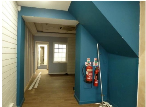
Rear of ground floor interior with stairwell and view to original south external window
