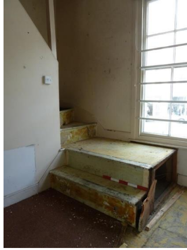
Carpet , metal nosings and side plywood panel removed December 2019 [50cm scale pole]
