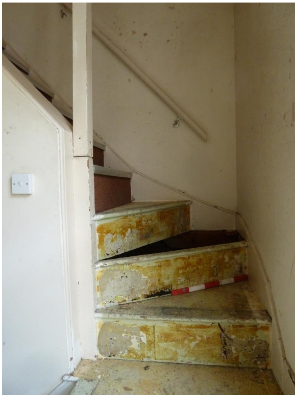
Three winder treads/steps followed by a steeped raked straight run of eight risers. [50cm Scale pole]
