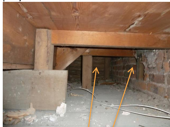
Original 19 th lath & plaster wall seen under the platform, RH Front elevation brick wall
