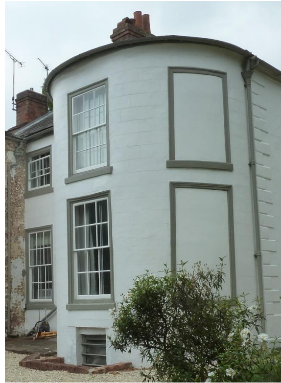
Bow bay ;painted ashlar effect stucco; flat lead roof with two full height 6/6 sliding sash windows; beneath semi basement window to cellar
