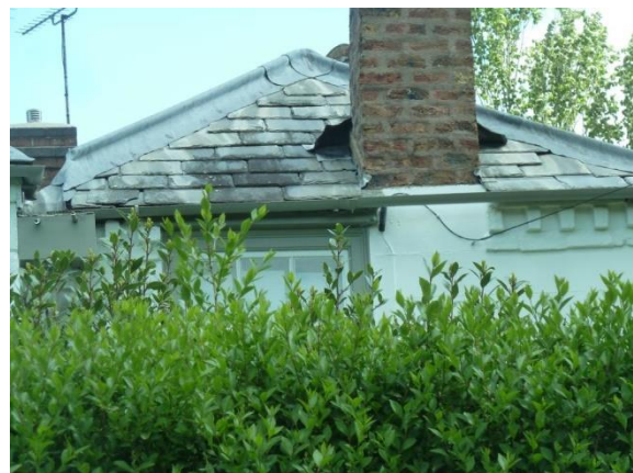
Brick clay tiled building that has been faced with ashlar effect stucco render and has one hipped roof covered in slates
