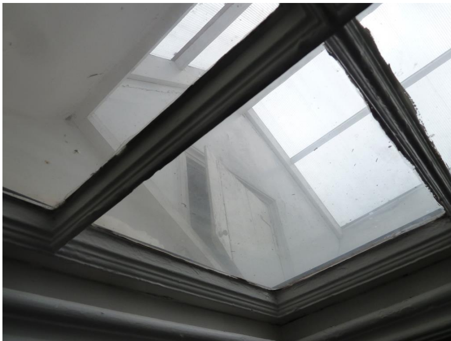
Fixed 4 light timber glazed trap door; attic space having access via a timber door with L hinges
