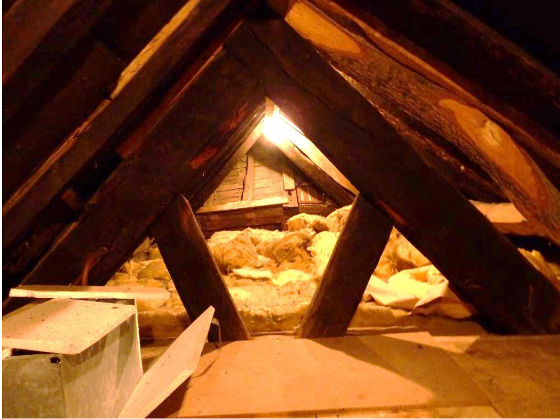
Soot encrusted Blackened Timbers
