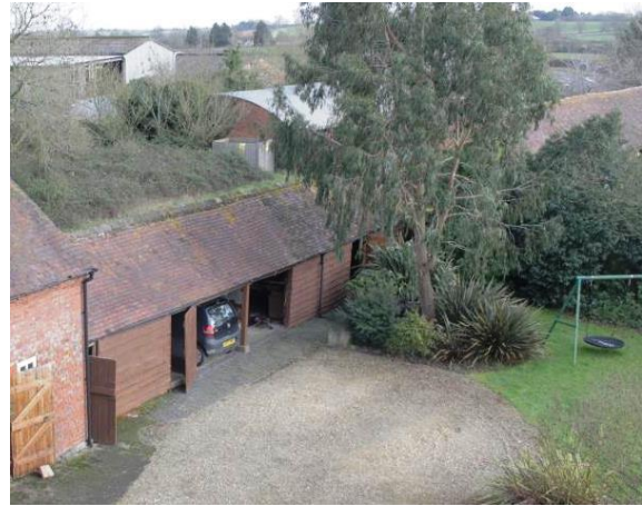
View External Elevations from Yard South; Single storey cow house/Shelter Sheds portioned and open and now part weather boarded, supported on posts.
