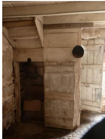
A: Door and Cupboard under loft stair; hanging board for harness, missing the pegs back of stable door
