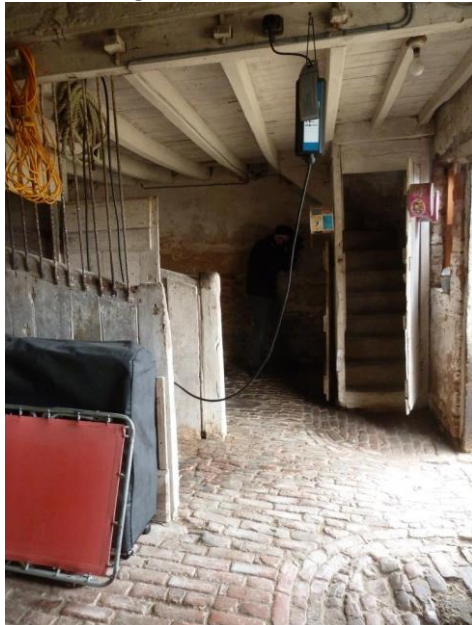
A: Staircase to loft; loft floor joists with through (tusk) tenon with face pegs
