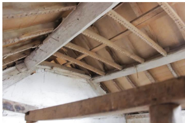
B; Principal trussed purlins. The lath and plaster ceiling has been removed
