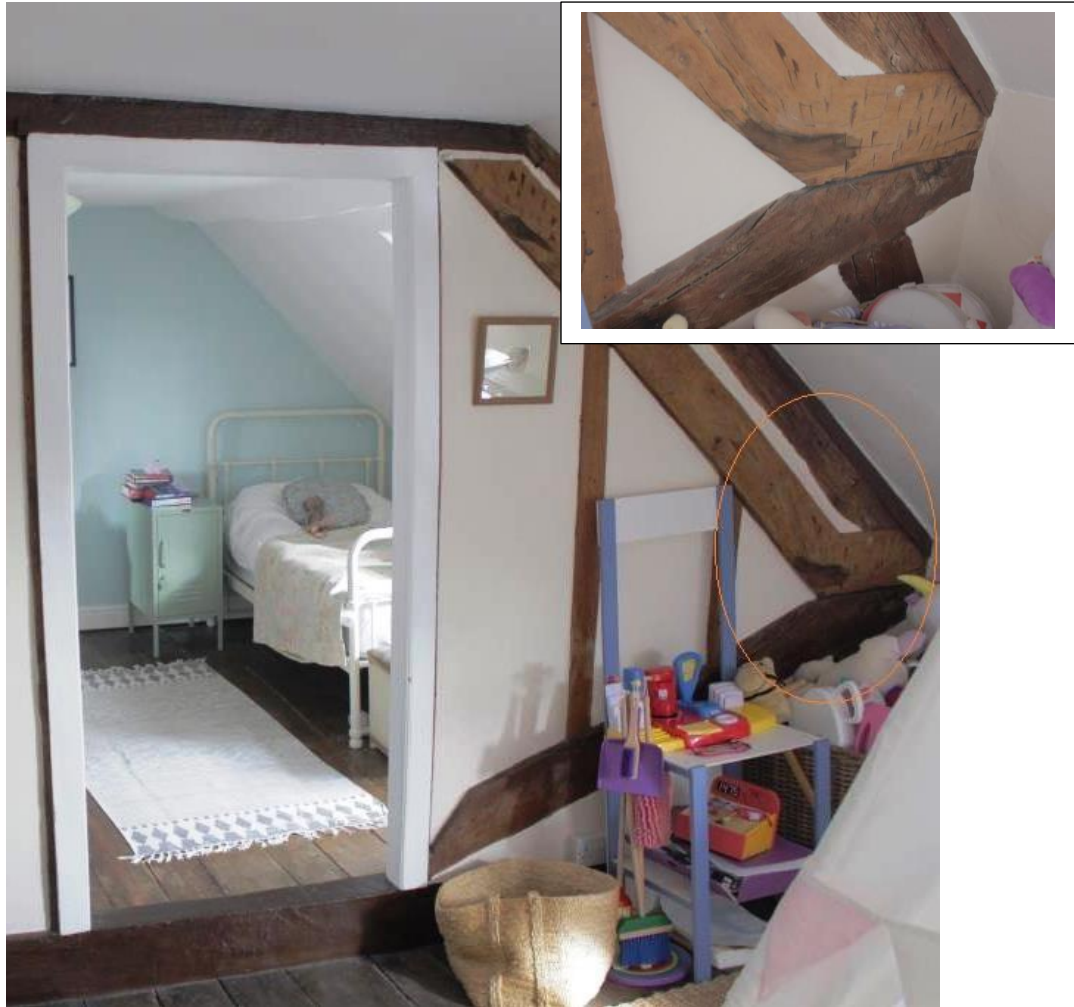
C18 Infilled vertical timber frame to truss to Bedroom 5; unusual unique double principal rafter, the lower one with a cranked end sawn construction. Collar visible at floor level.
