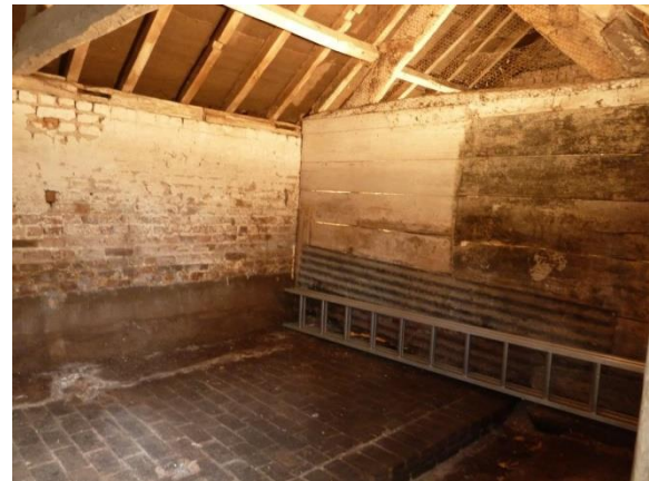
F : Roof Truss/ Dividing wall to G Flooring relaid late C19 C20
