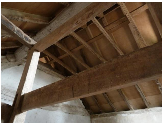
B; Loft Staircase rail; view to rafters and purlin; boarded with C20 Plywood sheets
