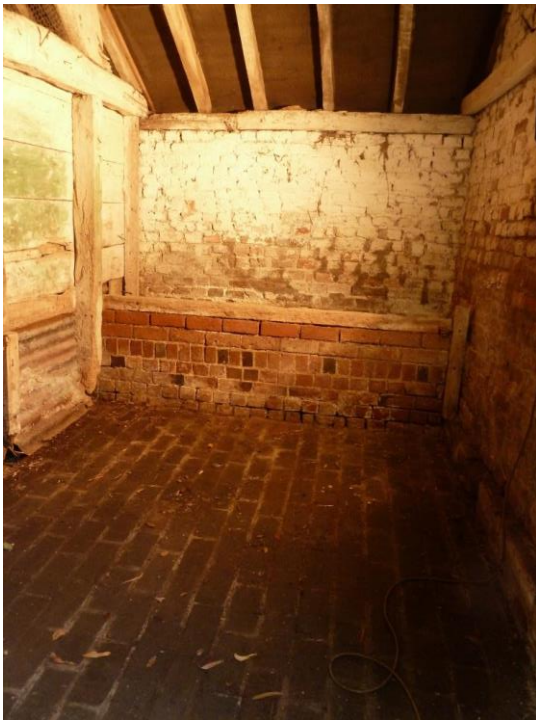
G: Brick trough with timber edge and example original timber bay division
