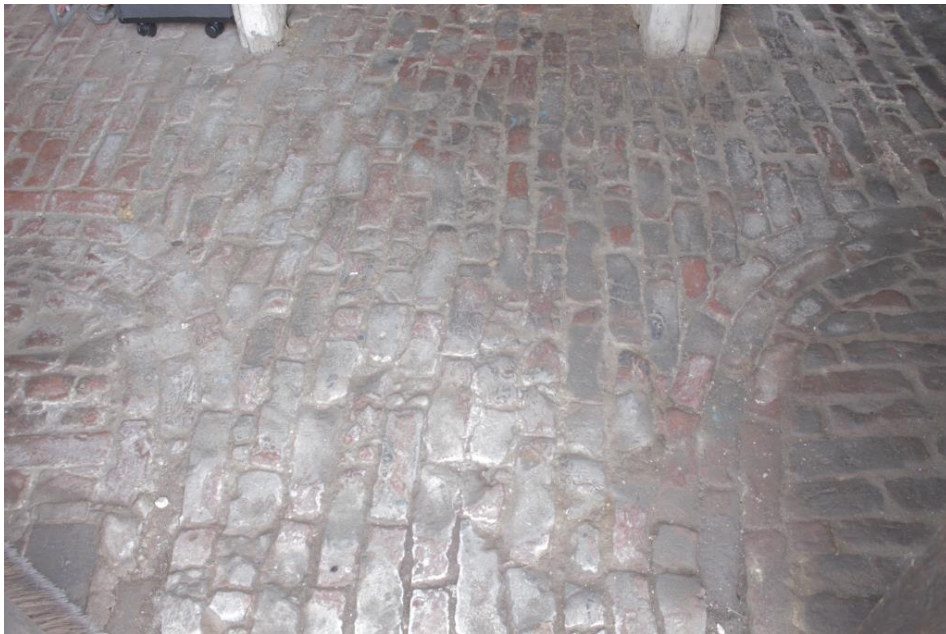
A : Pattern brick pavements well worn by horses hooves
