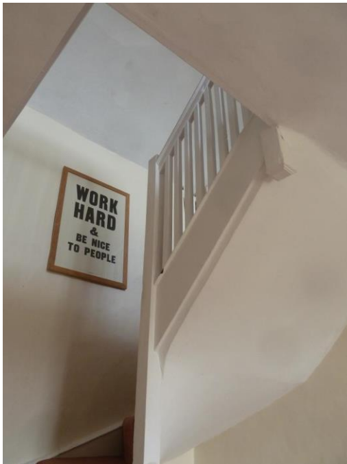
Underside of C18/C19 stairs are lath and plaster and structure is integrated into the plasterwork Description Bedroom 1
