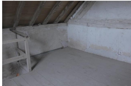
B; To S Front lime plastered ; Limewashed truss exposed rafters ; Pine boards, stable loft handrail
