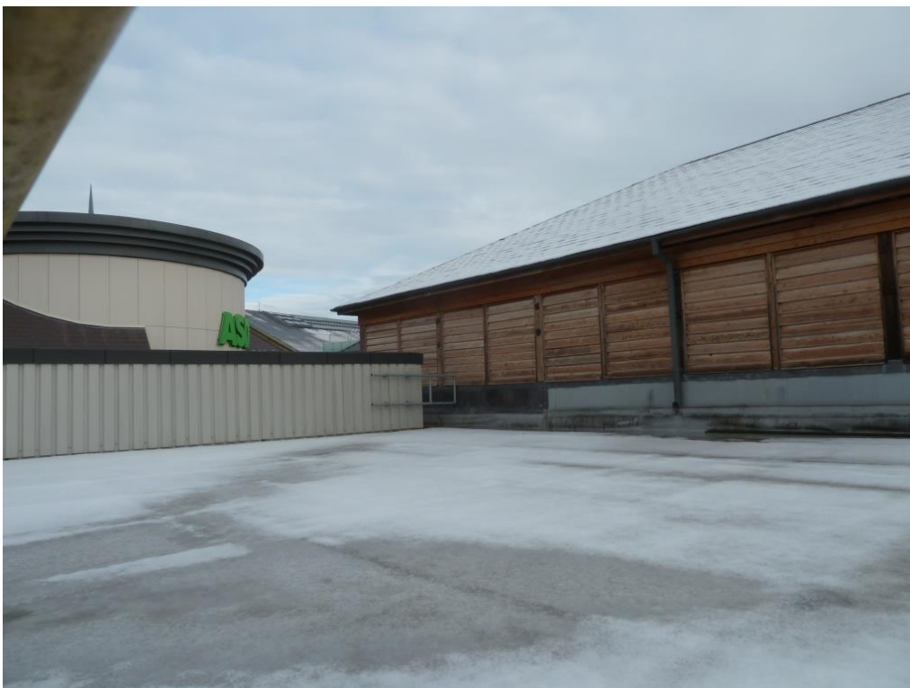
To the west end the new build attached up to the eaves; louvres visible above the new build roofline View seen from access hatch from new build to flat roof
