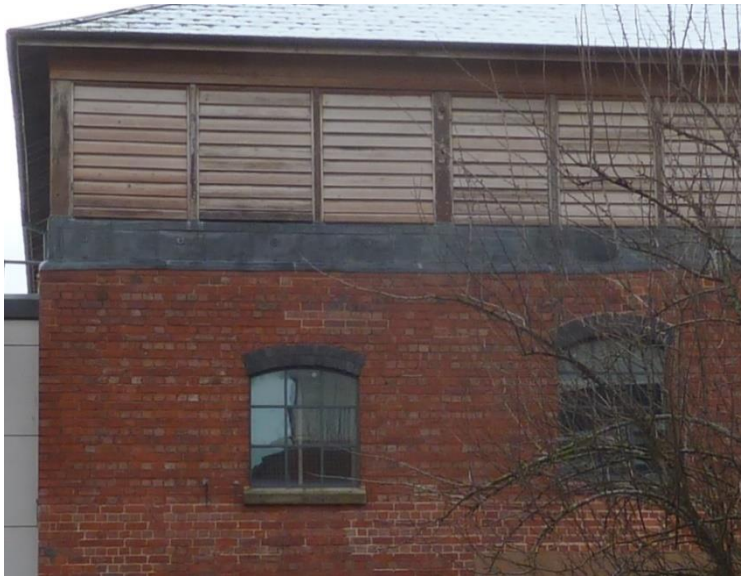
Restored fascia and existing refurbished louvres, x3 upper windows with blue brick arched lintels; stone cills
