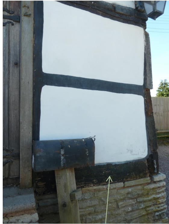
[Photo D] rendering to stone wall with horizontal black painted false timber. Timber sill probably a replacement
