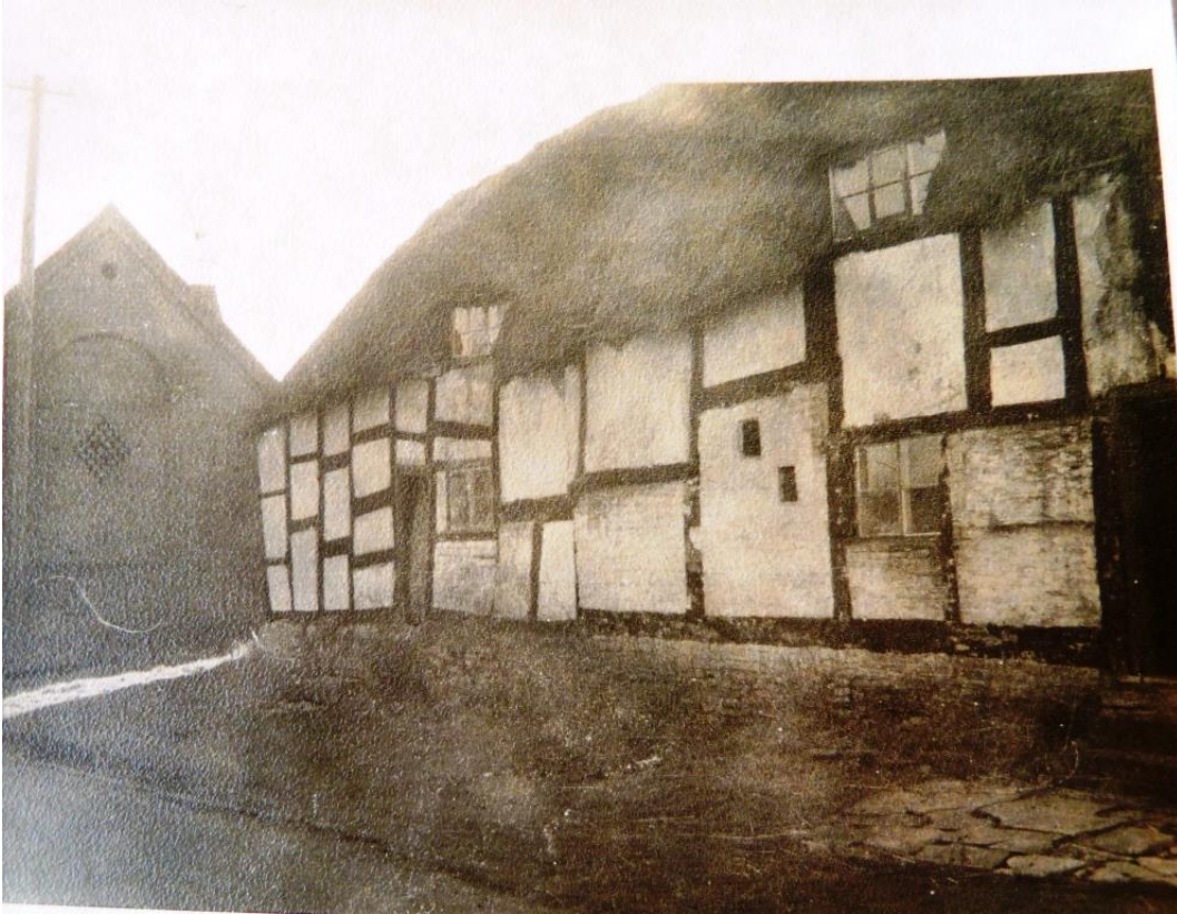
Analysis: View towards brick barn. Ground floor stone walling in panels and chimney stack with small fire window and end of bressumer beam visible.
