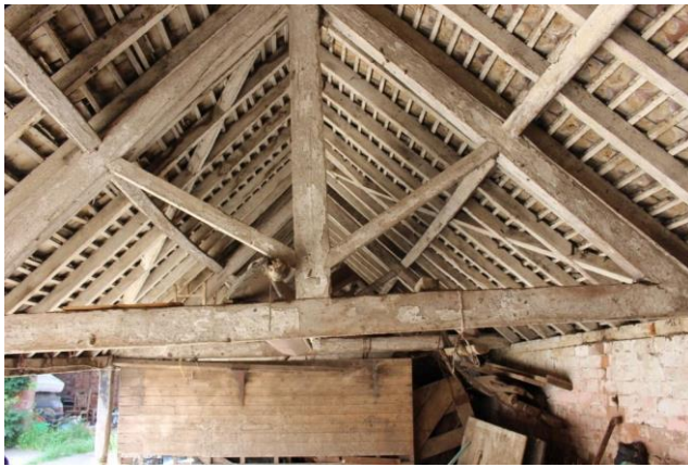
Roof structure [King post Baltic timbers] open Shelter Sheds X5 Bays X4 Trusses
