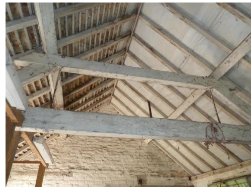
D: Roof truss interior space; diminished principal rafters and iron bolts passing through tie beam and collar for tension
