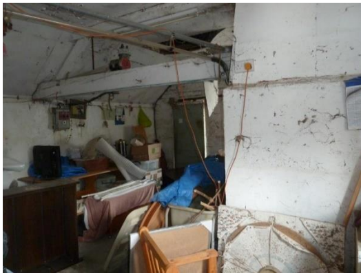
E: Interior space with roof truss and steel door to road, and breeze block and boarded store F
