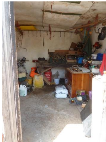
B: Workshop interior space; concrete floor hard board ceiling rendered brick walls
