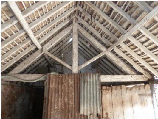
A: Side Entrance to former milking parlour at gable end Corrugated steel sheet and door enclosed in bay section with king post roof truss
