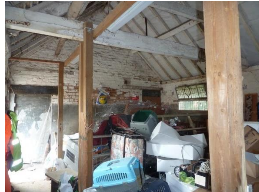
D: Interior former milking parlour looking to brick internal wall to west
