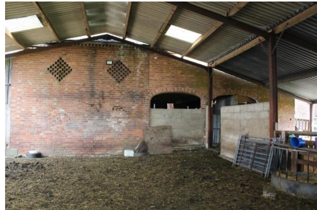
Rear of Hay barn with x2 brick archways[See Historic Photos 4.5] below former Granary probably for loading wagons
