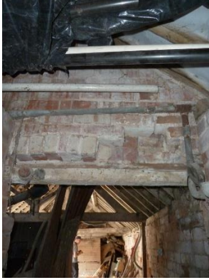
C: side entrance from shelter shed space A to former milking parlour with section brick relieving arch and timber lintel
