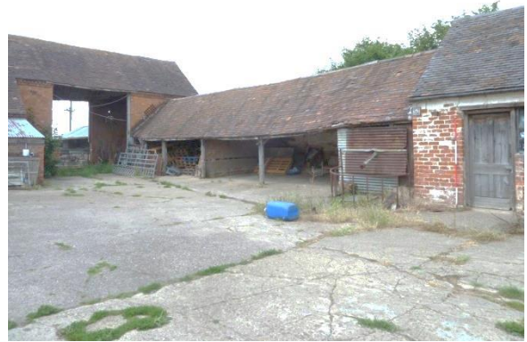
Range of open Shelter Sheds attached to Hay Barn [left] and former Milking Parlour [right]
