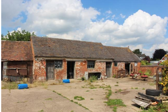
South elevation end section of shelter shed with corrugated iron sheeting to front; former milking parlour and adjoining feed room
