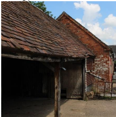
End section of shelter shed with covered bay for animal feed/chaff grinder and gable end of former milking parlour with brick coping at eaves
