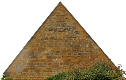
West elevation with stone gable copings and kneelers. Gable end has square panel 1832 datestone with initials W.H.
