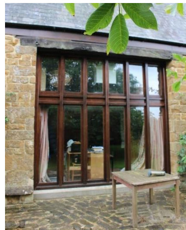
Window set in both sides of original threshing floor and former barn door entrance with reset post as lintel
