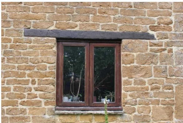
Detail south elevation casement windows; oak lintel stone; stone tile sill; regular coursed ironstone with quoins to side
