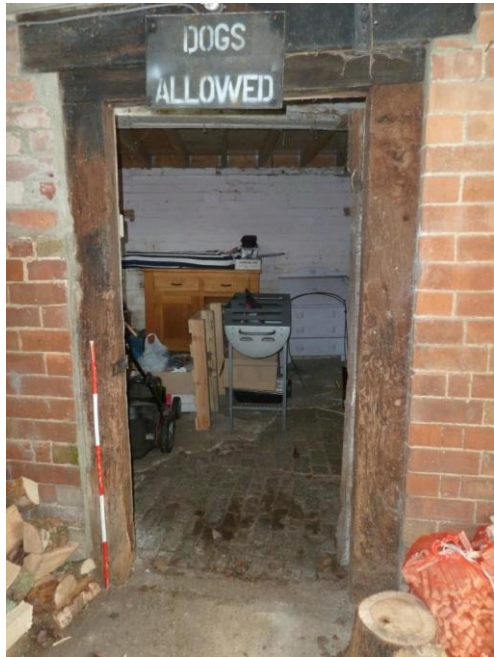
D Wide Elm doorframe/timber lintel [1m pole]
