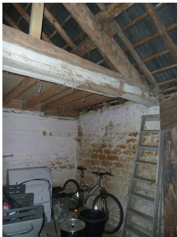
H Elm Roof Truss No 1 C19 Partition wall/ C18 Stone West wall. C20 timbers and boarding to roof.
