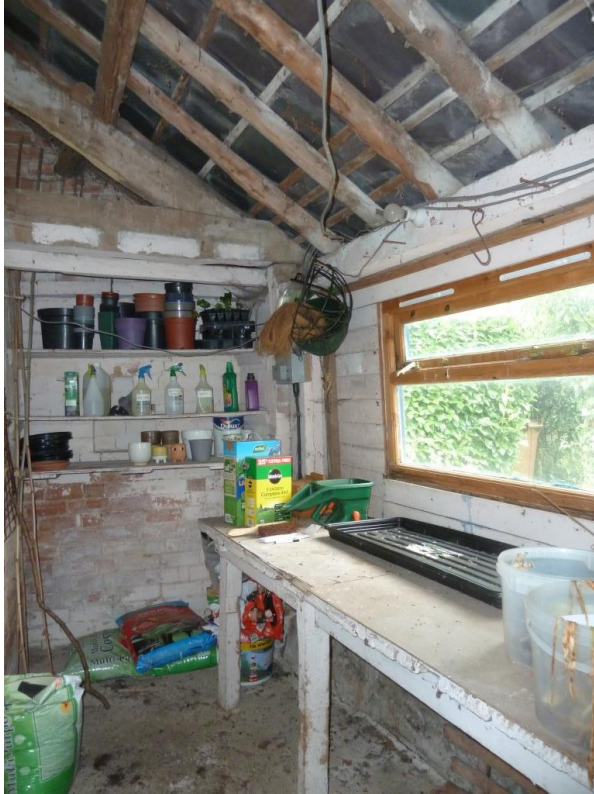
J View of Potting Shed; C18 Truss no 1 visible Front inside C20 timber cladding C20 window
