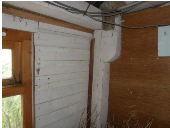
L C18 Timber Jowled painted post Truss No 2, C20 plywood boarding to C20 created lobby area
