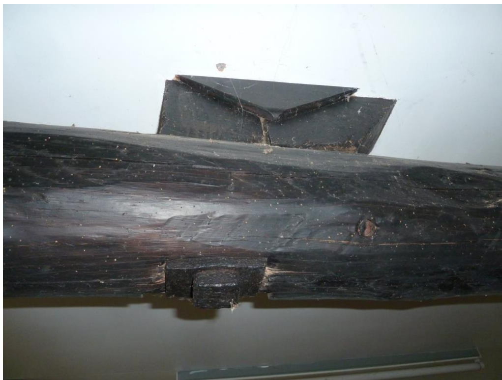
R Detail of central kingpost indicating mid /late C18 of truss No 3; bolted with iron tie to C19 pine horizontal; no C17 or earlier carpenters marks.
