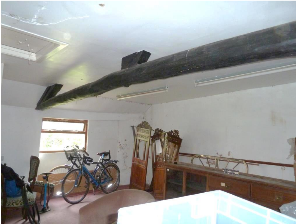
O View of Studio Room Timber Elm Truss No 3; horizontal beam later of C19 pine visible; but no posts; maybe hidden behind C20 boarding Loft access hatch but not able to be opened so no access made. Floor carpeted
