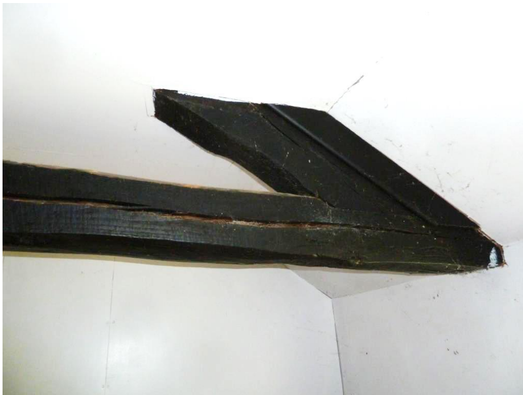
Q Detail of elm timber Truss No 3; horizontal beam pine; and surrounding C20 boarding
