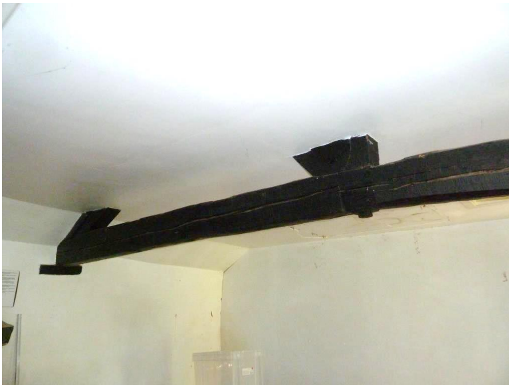
P View Of C18 elm Truss No 3; ceiling boarded; no access to roof space
