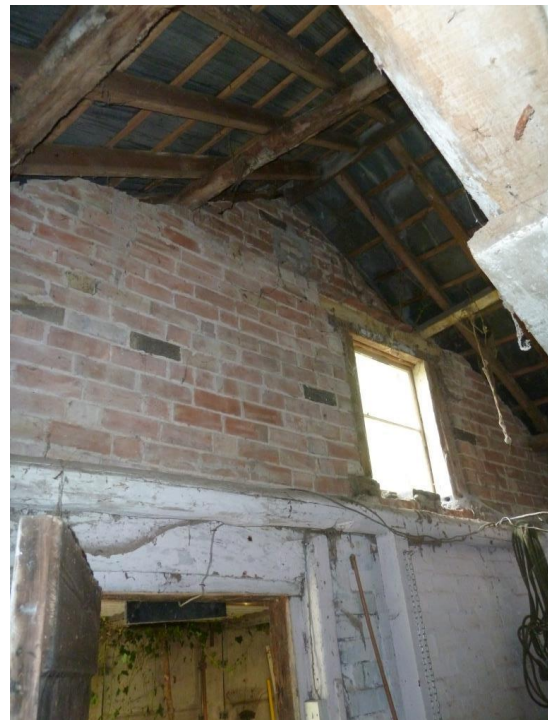
F Inside of C19 brick gable walling and inserted C19 window opening
