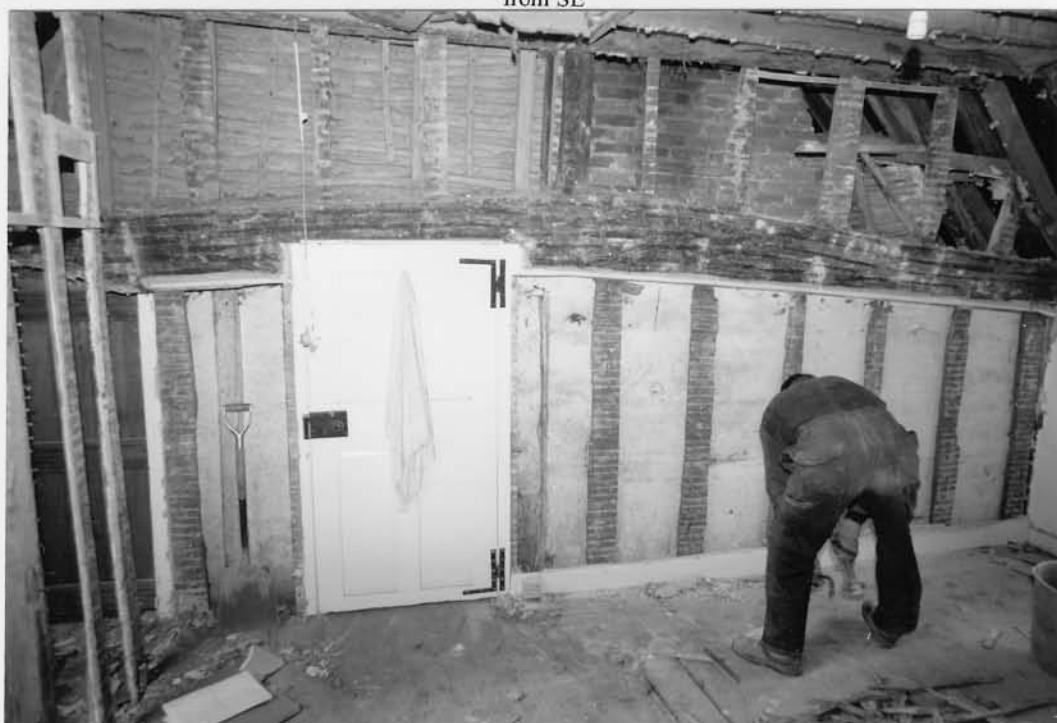
Plate 6: First floor, showing central beam spanning hall, with panelled door with L-shaped hinges inserted, stack behind and to right, from N
