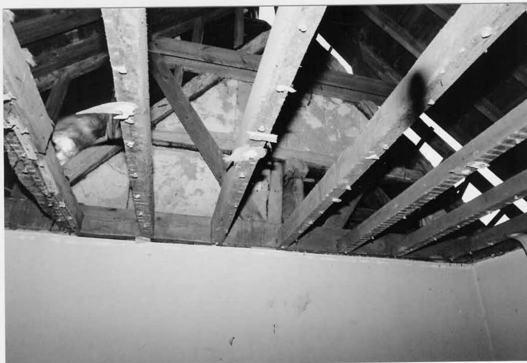
Plate 8: Closed roof truss at north end of hall from inside NW wing, showing sawn off through timbers, from NW
