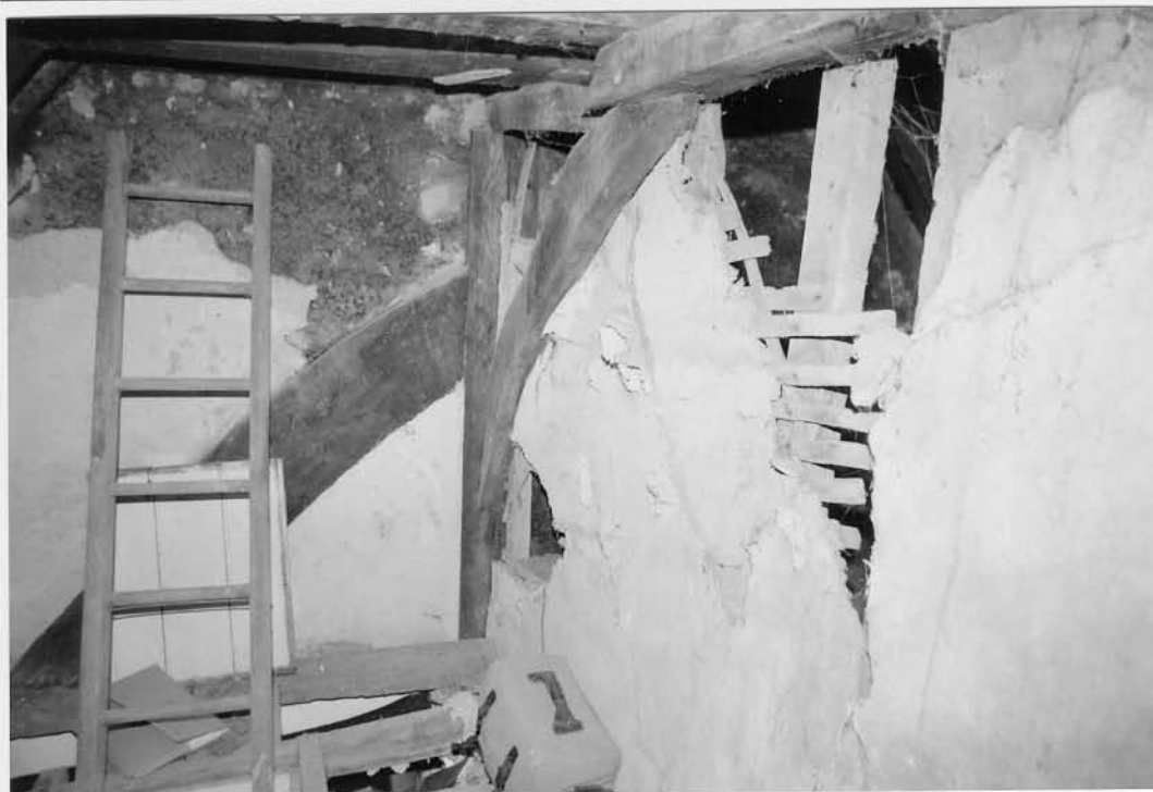
Plate 7: Braces in roof at southern end of hall showing closed truss from N
