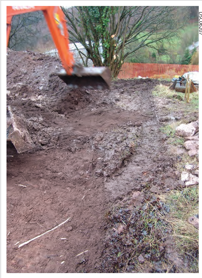
Plate 09: View along former access track to the south east during surface removal prior to path construction [102] exposed
