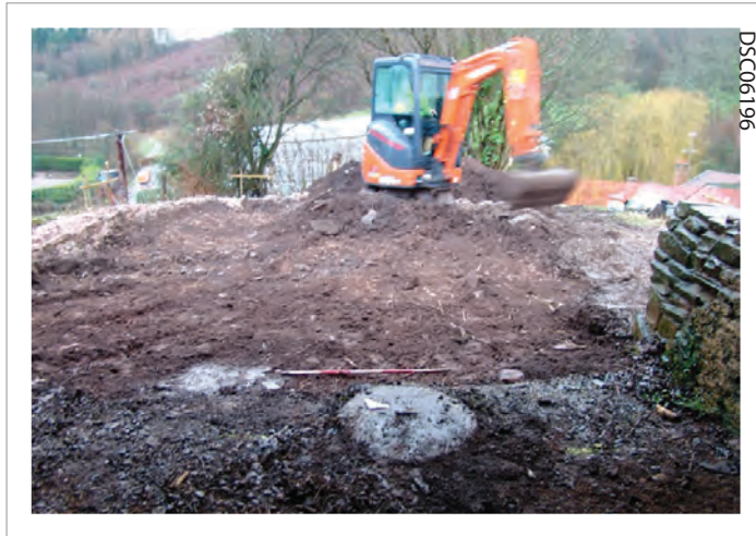
Plate 05: View across site from covered north west end, Concrete post foundation in foreground (not a mill wheel)
