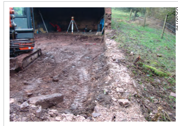
Plate 04: View along north east wall showing debris removal internal and soil build up external
