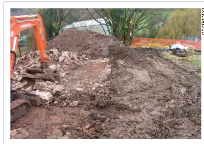
Plate 08: View along former access track to the south east during surface removal prior to path construction. 2
