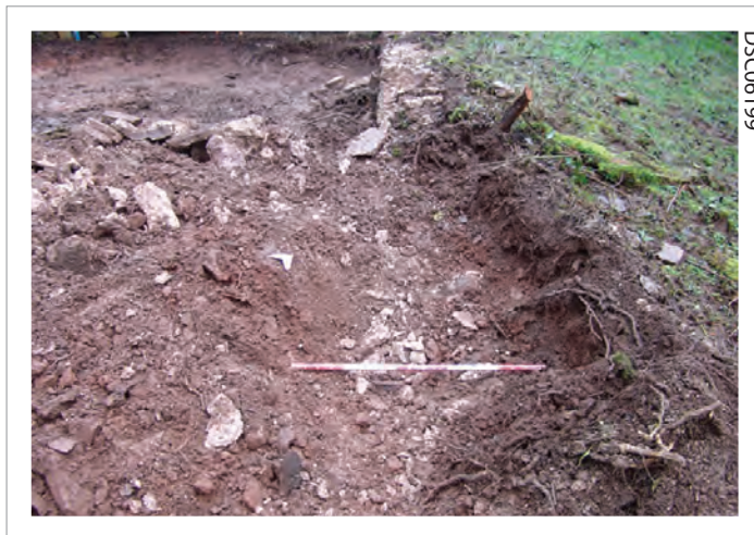
Plate 07: View along north east wall showing debris removal internal and soil build up external and depth of foundations
