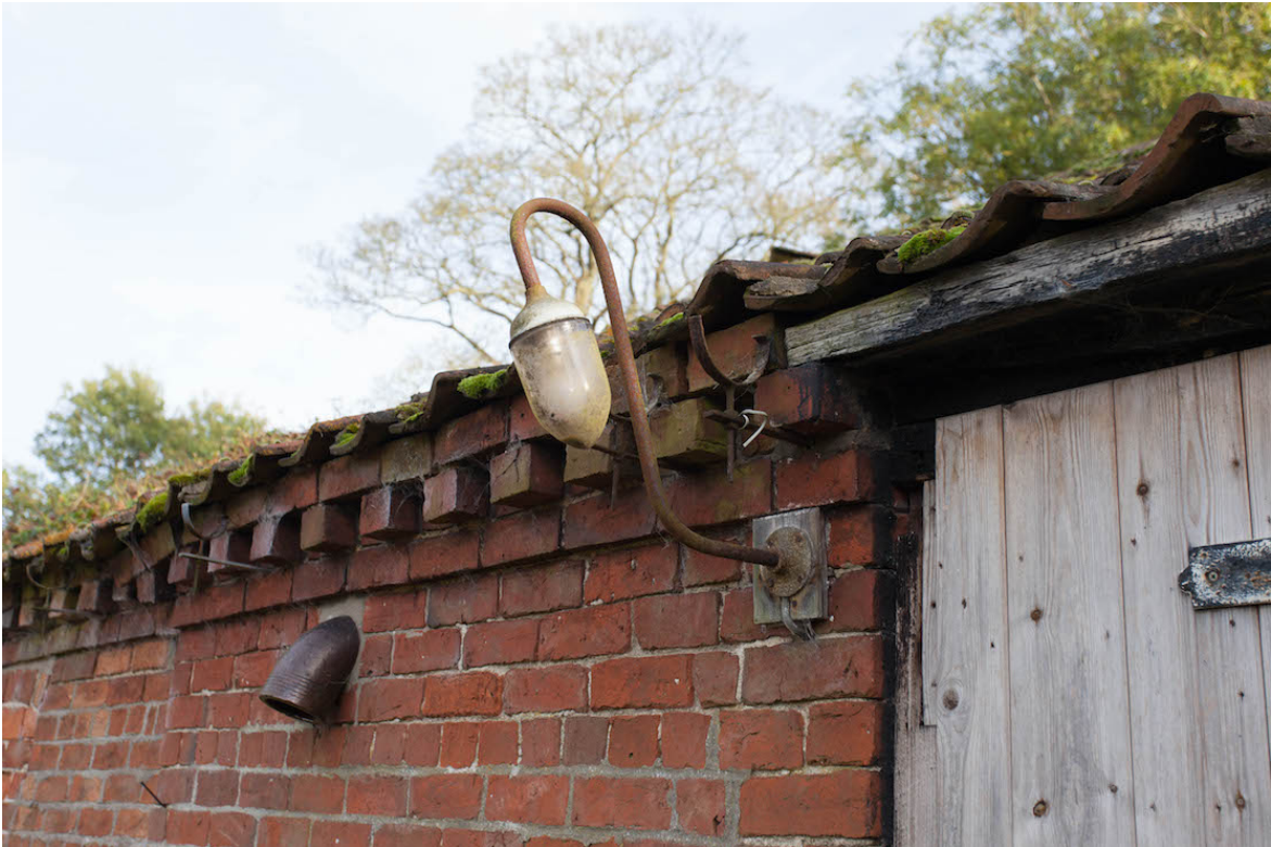
Plate 33 (shot 48) – Exterior of southern section of north western elevation showing modern light fitting, iron rainwater fittings and reused drainage pipe set into wall assumingly for ventilation, looking east.
