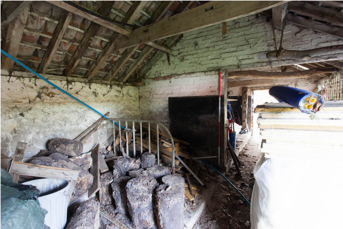
Plate 21 (shot 34)– Interior of southern section showing galvanised cattle dividers, looking south west.
