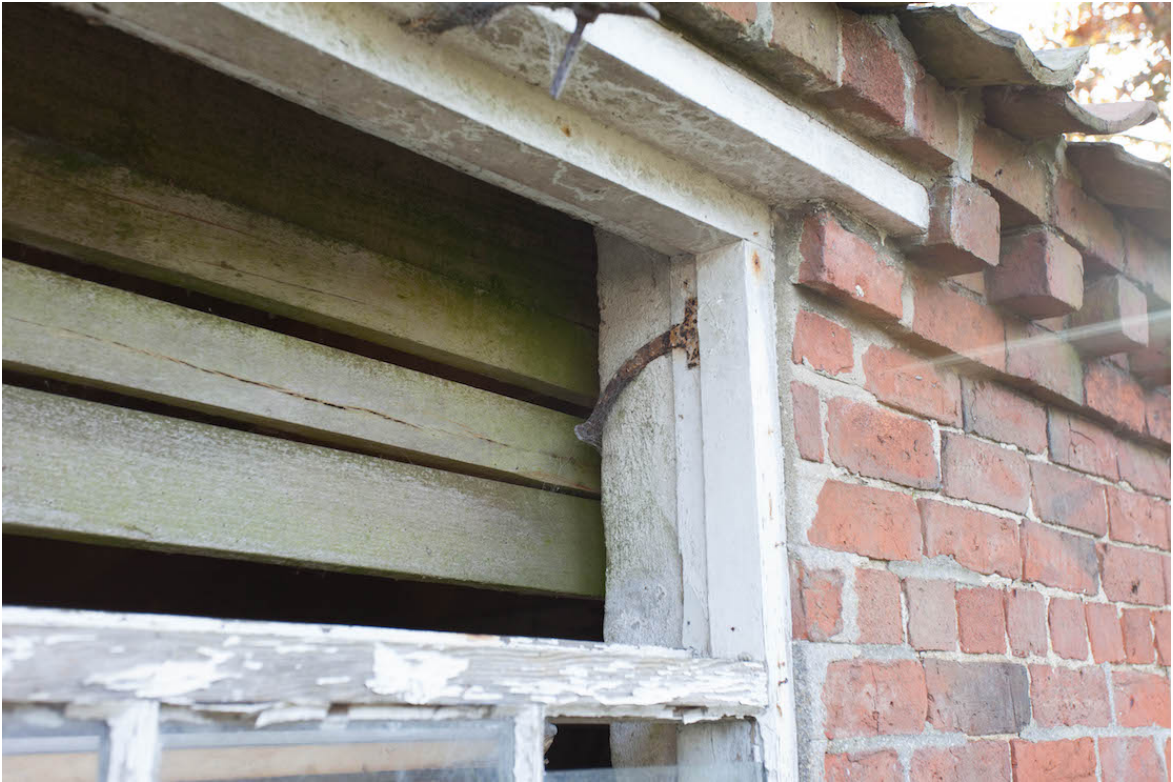
Plate 31 (shot 46) – Exterior of southern section showing missing upper ventilation casement in large window, looking south.
