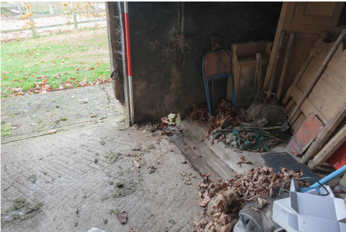
Plate 22 (shot 35) – Interior of southern section showing modern concrete floor with gully, looking north.
