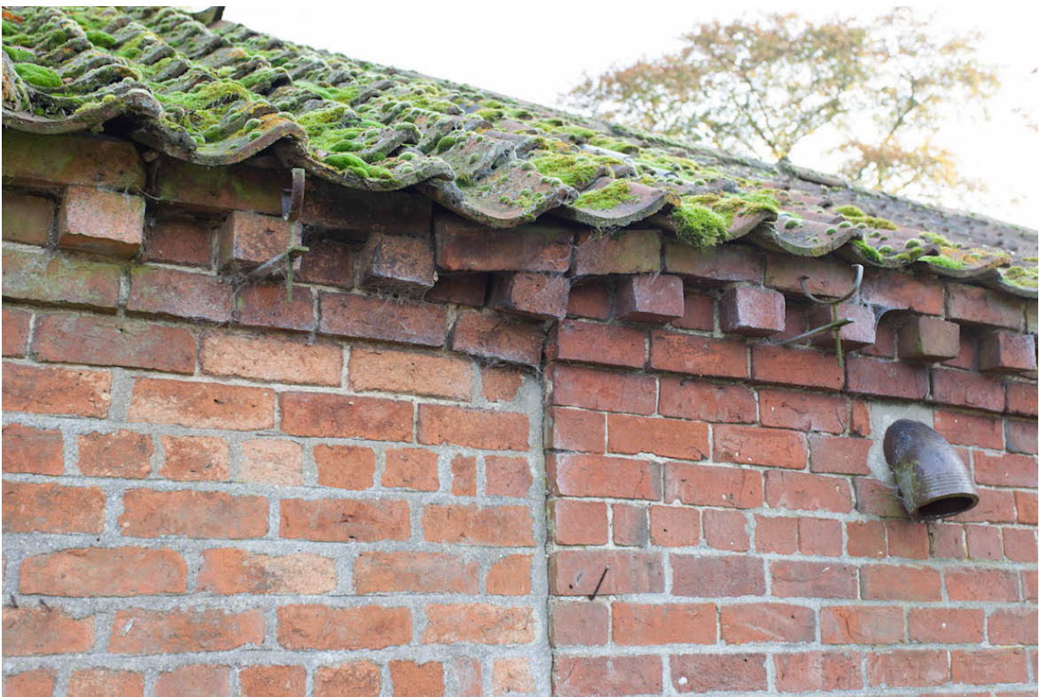
Plate 32 (shot 47) – Settlement at join between northern and southern sections, looking south.
