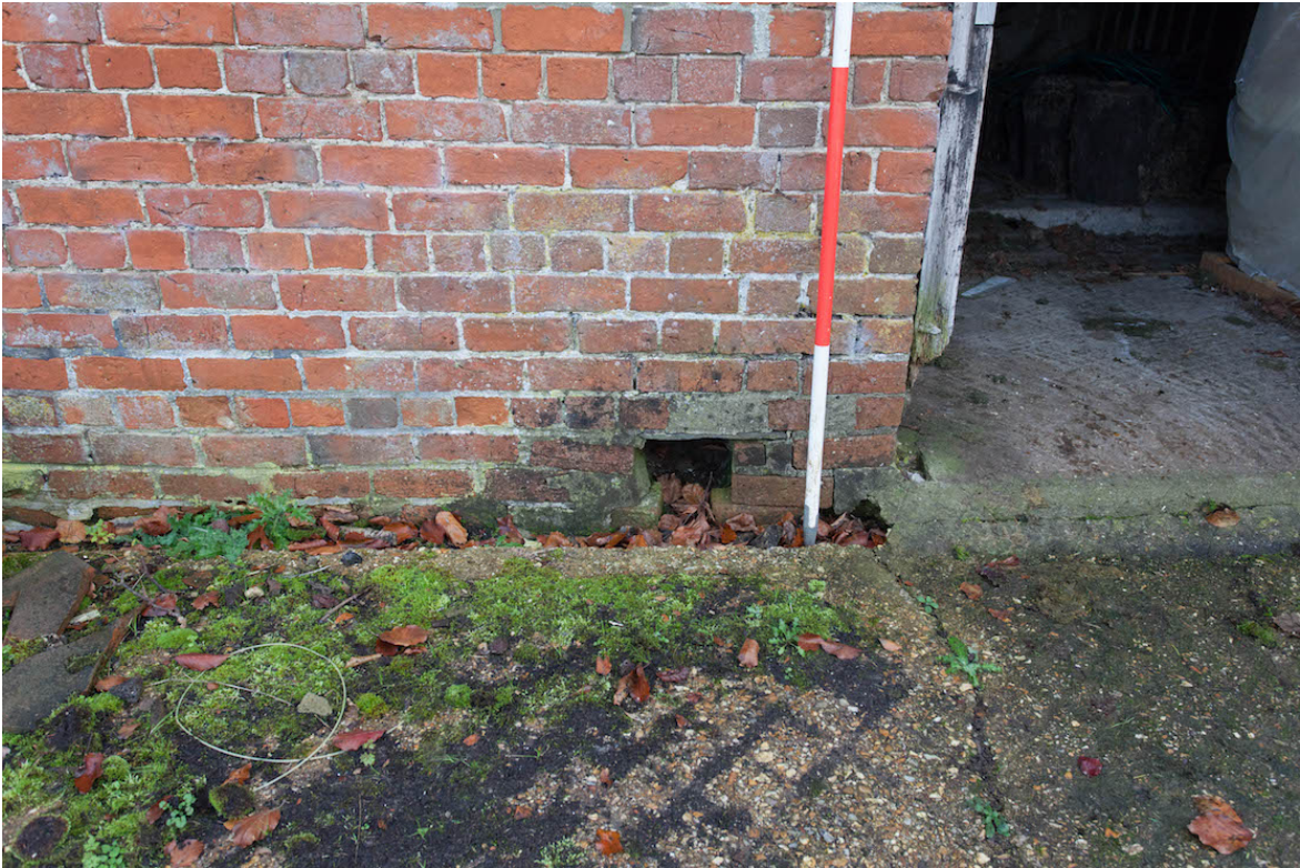
Plate 23 (shot 36) – Exterior gully opening in southern section of north western elevation, looking south east.
