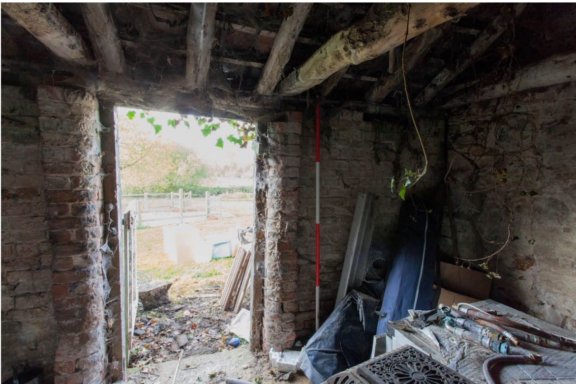
Plate 30 (shot 45) – Interior of northern section showing reinforced brick door pillars, looking north west.
