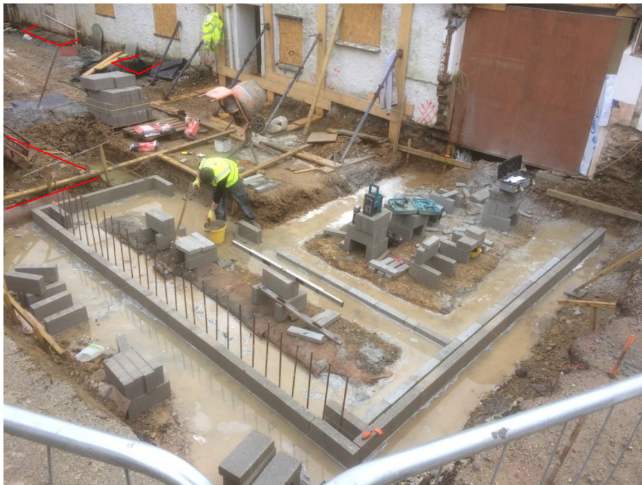
Figure 3. Area to the north-west (rear) of farm house during construction. area watched from excavation to start of building work.
