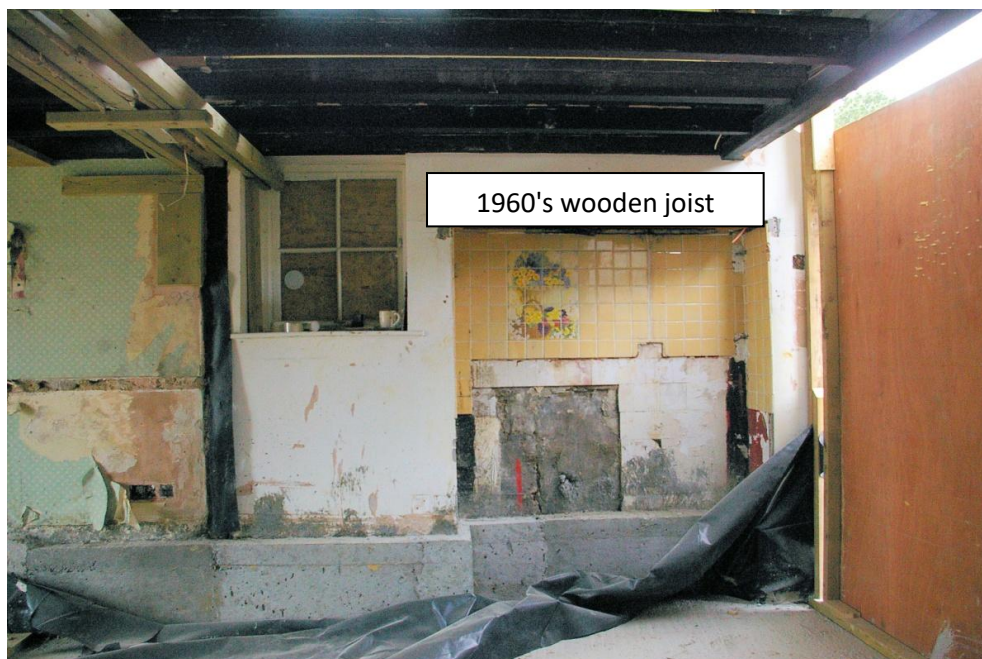
Figure A2.7. A fireplace in the kitchen area for Aga [1960's?]. (Author 2017).
