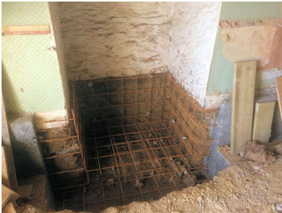
Figure A2.9 Fireplace with the base removed to reveal its construction. (Lilly-Lewarne: Aug 2017).
