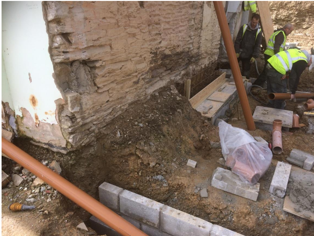
Figure 4. Area to the north-east (side) of farm house during construction. area watched from excavation to start of building work.
