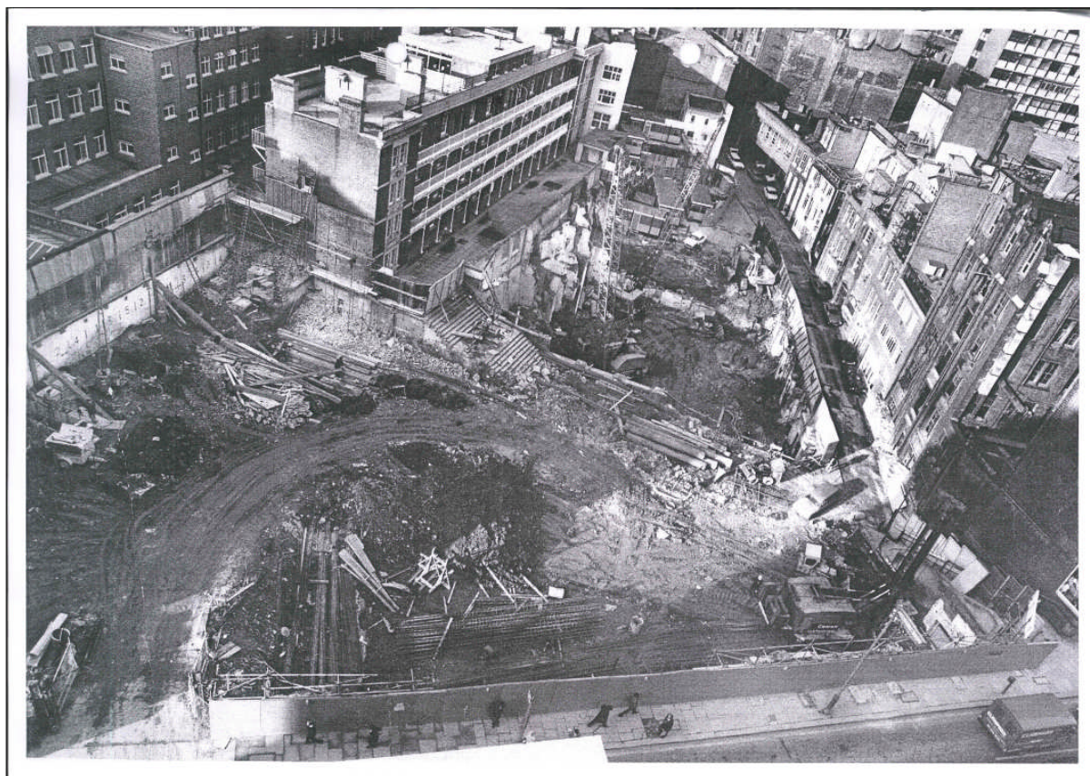
Plate 1. Photograph taken during the construction of the current building in the mid 1970s looking north from Charterhouse Street (Source unknown).
