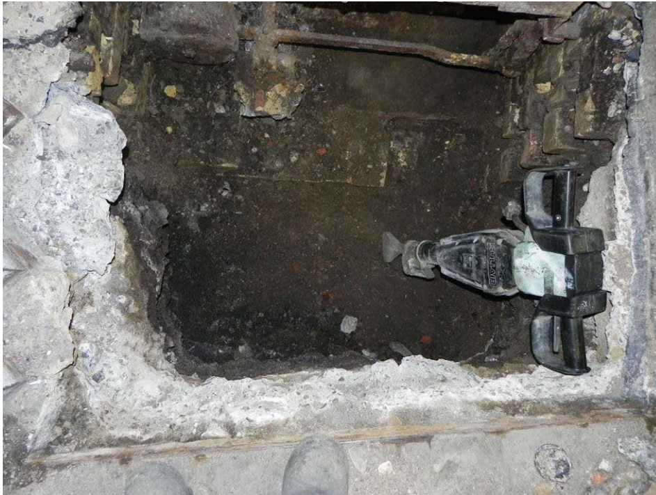
Photo 19: Railway Tavern Trial Pit- Foundations of the Railway Tavern with 19th-century walls, disused machinery, and construction backfill (north at top)
