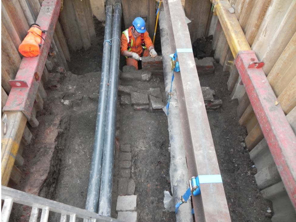
Photo 4: Trench 1 – Post-medieval brick structures, including wall [325] (left), drain [321] (centre to centre right), wall [332] (top), floor [329] (centre bottom) (looking east).
