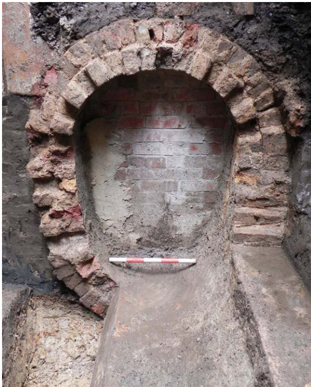
Photo 7: Profile of sewer [535], backfilled and bricked up westward, and largely broken out within the trench (looking west).
