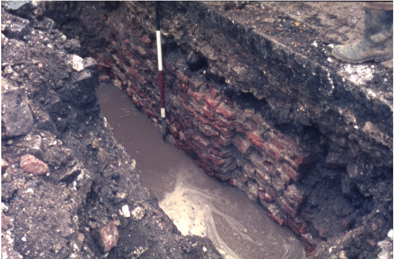
Pl. 8. Part of the Town Wall exposed in a machine trench during building work in Humber Street in 1973. This appears to be running alongside the edge of the pavement. Some 14 courses of brickwork were visible in the two surviving slides, but, apparently up to 22 courses were recorded in some sections of the trench. [Photo: Peter Armstrong. Copyright Hull Museums.]
