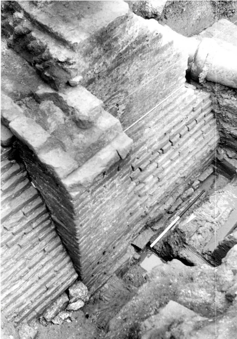
Pl. 18. Beverley Gate, 1986. An oblique overhead view of the junction of the medieval Town Wall (to the left) with the north-west corner of the 17th-century Guard Chamber; there is a butt joint, where the Town Wall has been cut back to form a clean vertical face against which the new corner buttress can be built. The pronounced external batter of the lower sections of both the Town Wall and the Guard Chamber can be clearly seen. [Photo: Humberside Archaeological Unit]
