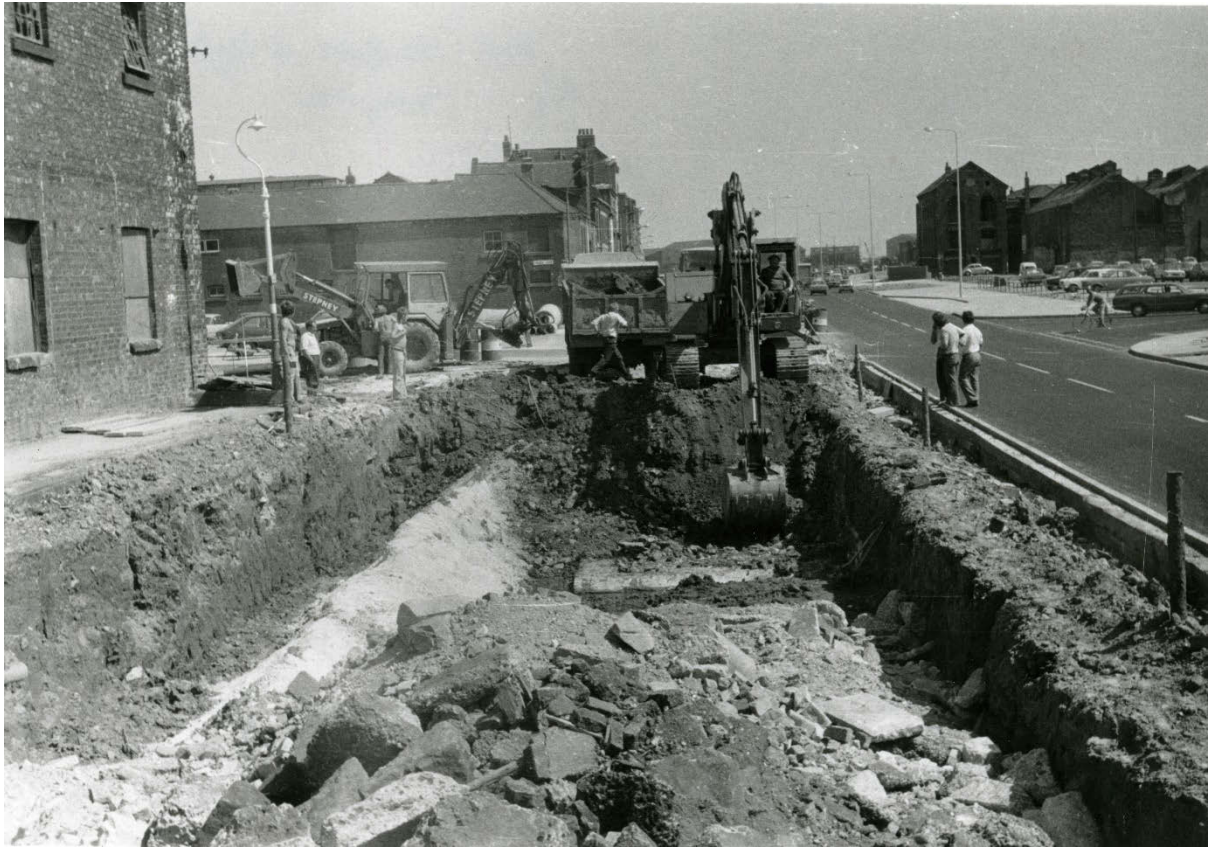
Pl. 9. A machine uncovering the remains of the Myton Gate in July 1976 in the course of building what is now the dual carriageway of the A63 Castle Street; viewed from the west. The footings of a counterweight pit, in front of the Gate, can be seen beginning to emerge. The brick walls of the Grade II Listed Warehouse no. 6 can be seen on the left, with the entrance to Prince's Dock Street just beyond; in the right middle ground (considerably beyond the machine) can be seen the junction of Humber Dock Street with what is now the south carriageway of Castle Street. [Photo: Humberside Archaeological Unit.]
