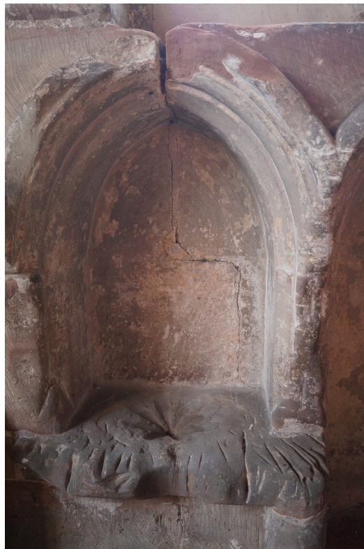
Plate 4. Damaged sedilia in Lady Chapel noted by Pevsner.
