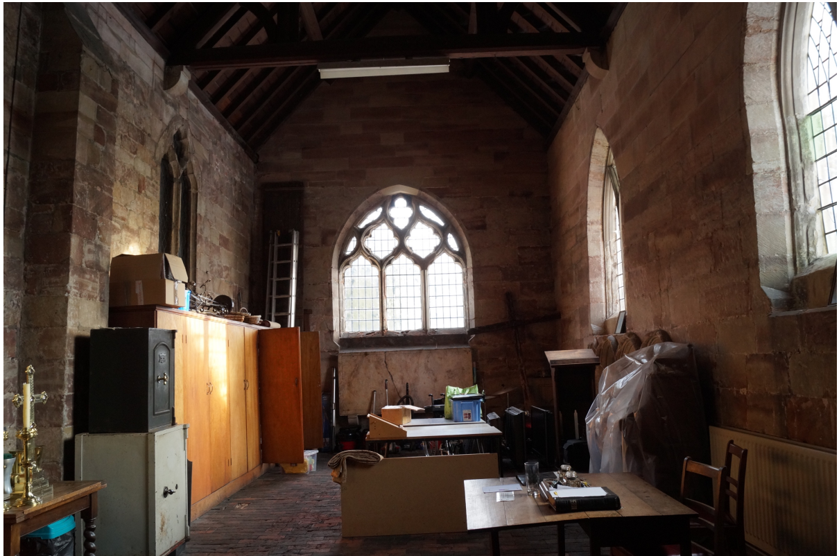
Plate 19. Overall shot of the Lady Chapel revealing how subdivision would detract from its architectural integrity.
