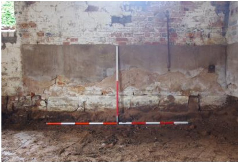
Plate A Construction layers and foundation sequence in Room 1 Range 1 looking northwest.
