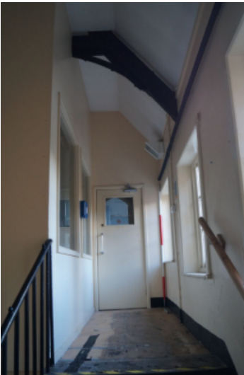
Plate 34 First floor landing showing modern additions/alterations, an original hammer beam truncated by modern partition wall. 82
