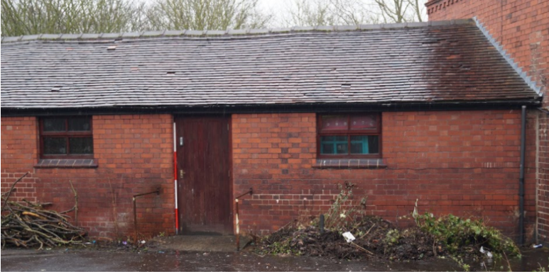
Plate 93. South west (front) elevation of the ancillary building which was used as cloakroom and washroom.
