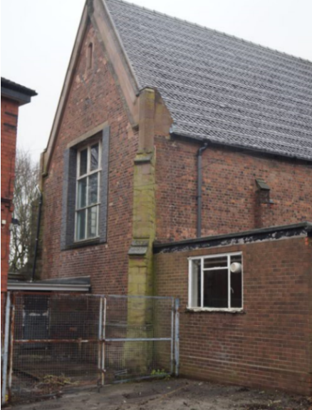
Plate 69. View of north west facing elevation of mid-19 th century main hall showing detail of sandstone buttressing and blue brick window jambs..
