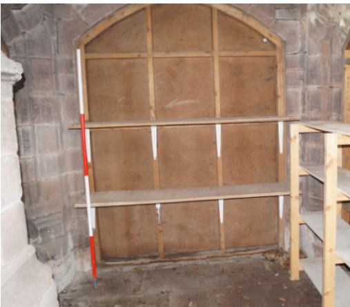
Plate 12. Detail of blocked archway in porch. The arches in the porch were originally open. 21, 22
