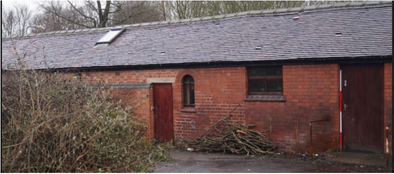
Plate 94. South west (front) elevation of the ancillary building showing detail of windows and doorways. To the left the Edwardian phase of the ancillary building adjoins the 1970s extension.
