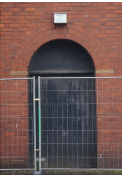
Plate 92. Detail of brick arch doorway above which leads into the entrance to the boiler room.
